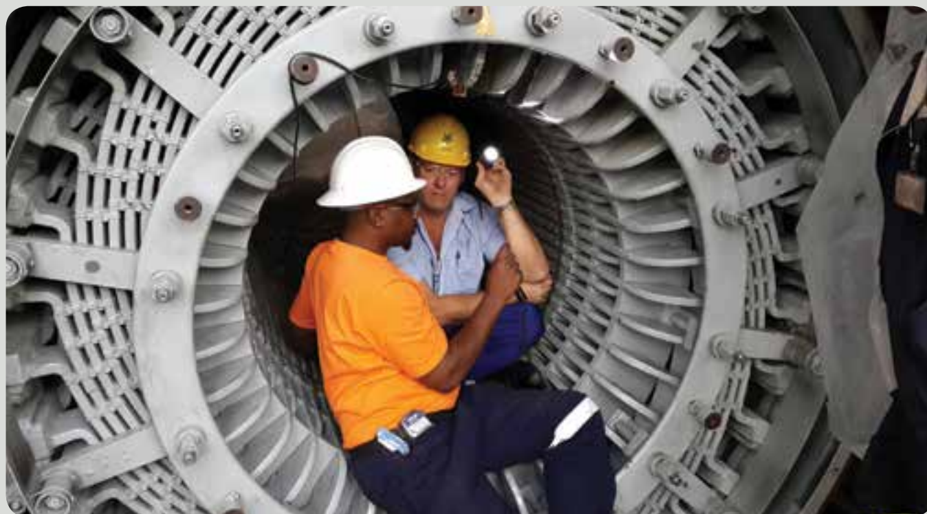
Marthinusen & Coutts' divisional CEO Richard Botton and senior artisan Shepherd Chigwa inspect the 60 MW generator stator at Kelvin Power Station prior to its repair. Over the past 18 months, Marthinusen & Coutts and ACTOM Turbo Machines have performed a comprehensive range of repairs and refurbishments for Kelvin Power Station in Kempton Park. Marthinusen & Coutts re-
