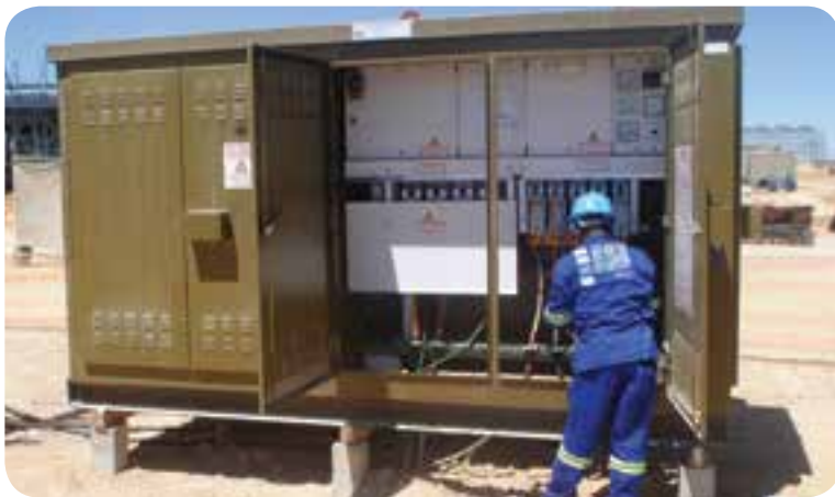
Terminating a distribution board at Enl Electrical's contract at Husab in Namibia.
