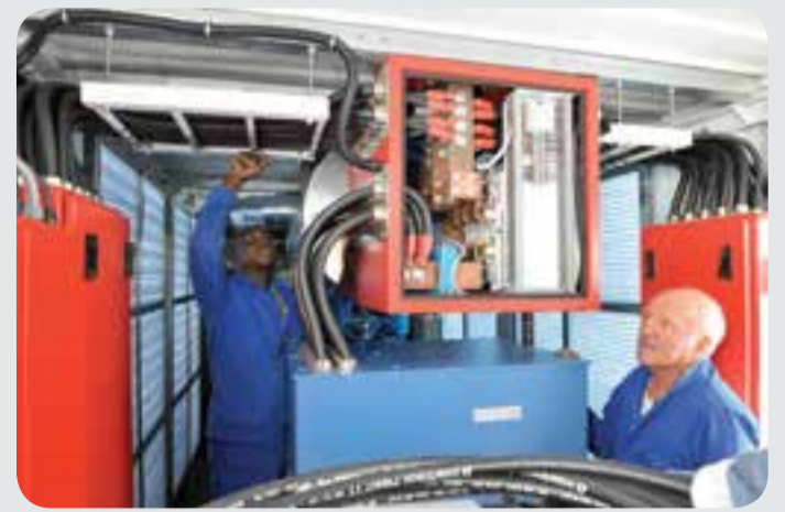
A view inside a containerised generator set from Zest WEG Group's Generator Set Division.
