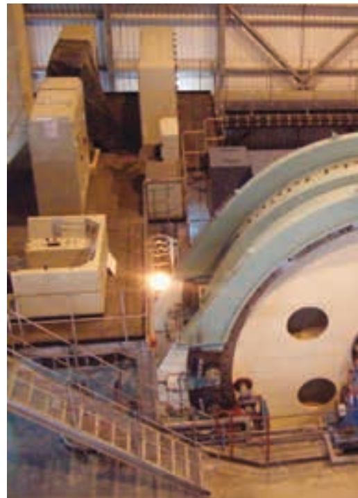
The FLSmidth 6.5 m Koepe Winders at Impala 16 Shaft showing the 90° orientation for space saving.
