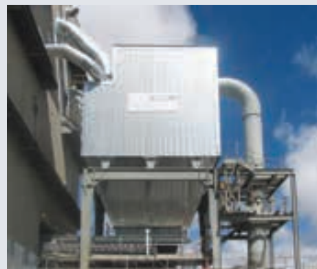
The bag filter John Thompson APC has been contracted to install at the De Hoek factory's Finishing Mill 6 will be similar to that shown above, which the business unit installed at PPC's Slurry factory's Finishing Mill 4 two years ago.
