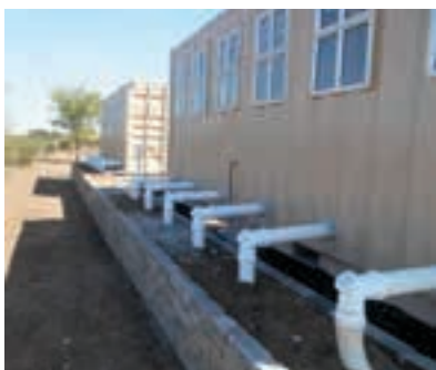
The new containerised flush ablution facilities installed by ThyssenKrupp at Mosima 2 Primary School in Lephalale 1.
