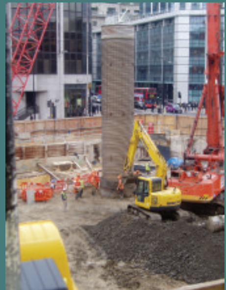
▲ Construction of London's new Heron Tower uses 16 threaded steel pile casing structures
