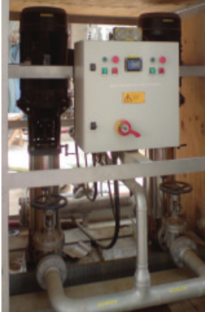
▲ Two 30kW high pressure pumps, plus control panel
