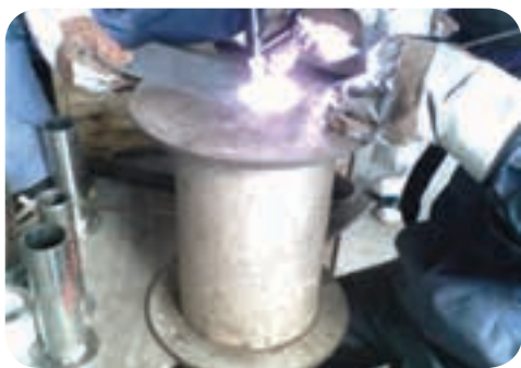
Figure 7. The welding of small diameter-connecting pipe and backing rings in the argon gas box.
