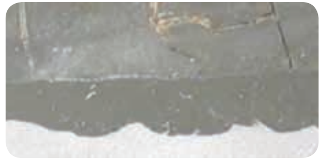
The crack on the right in this hard top surface layer of Fluxodur 58 TIC-O has been stopped by a Supranox RS 307 buffer (bottom) layer.
