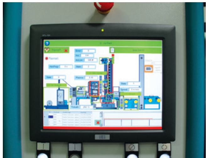
○ Figure 6: HMI with a touch-screen, user-friendly interface on PlasmaPREPLATE tinning line
