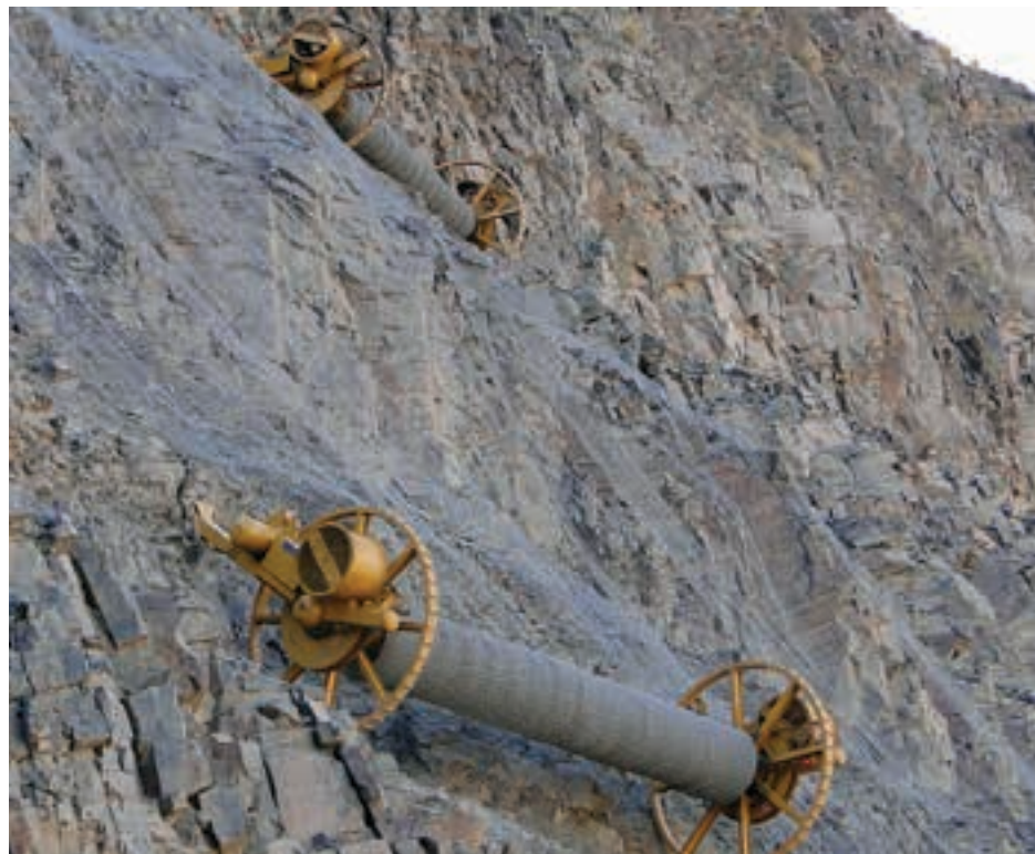
Two Decoilers specially designed for the project were deployed on the contract.
