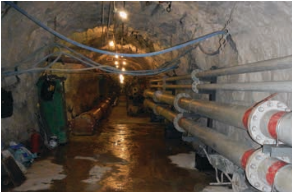
Access to 3 Shaft deepening and view of the installation of pump and water column which will assist with water management.
