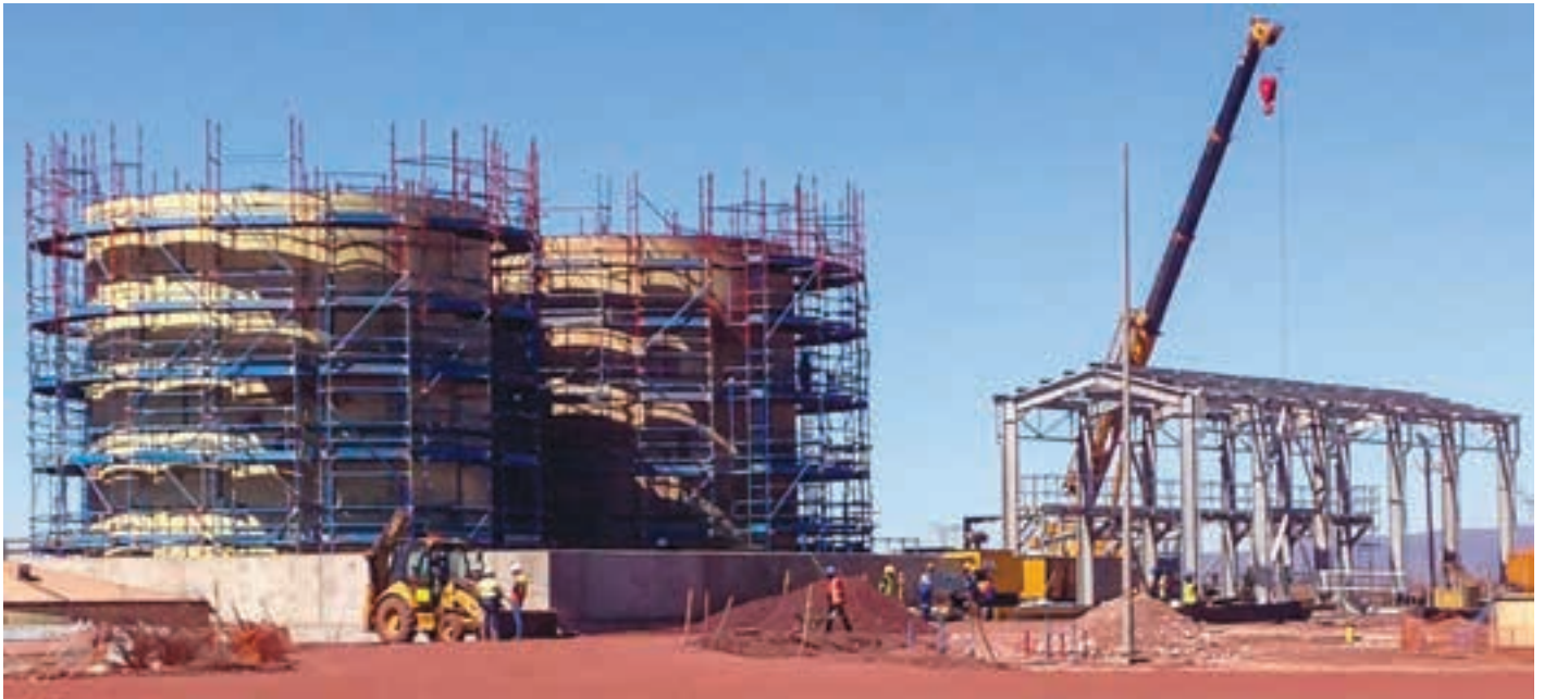
Sishen's new heavy mining equipment (HME) filling station under construction (photo: VBKom).
