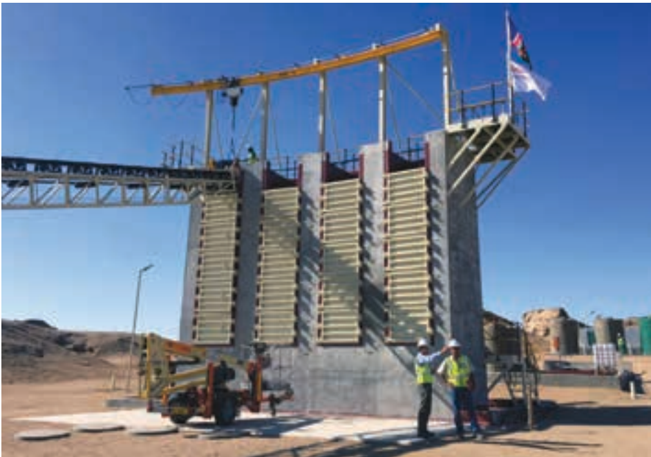
Acid leaching of agglomerated ore in the demonstration plant occurs in four 2 m x 2 m x 6 m leach cribs, seen here. In addition to the cribs, eight 5 m high columns with an internal diameter of 0,18 m enable parallel leaching (photo: Bannerman Resources).
