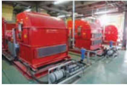
TOMRA XRT sorters installed at Karowe.
