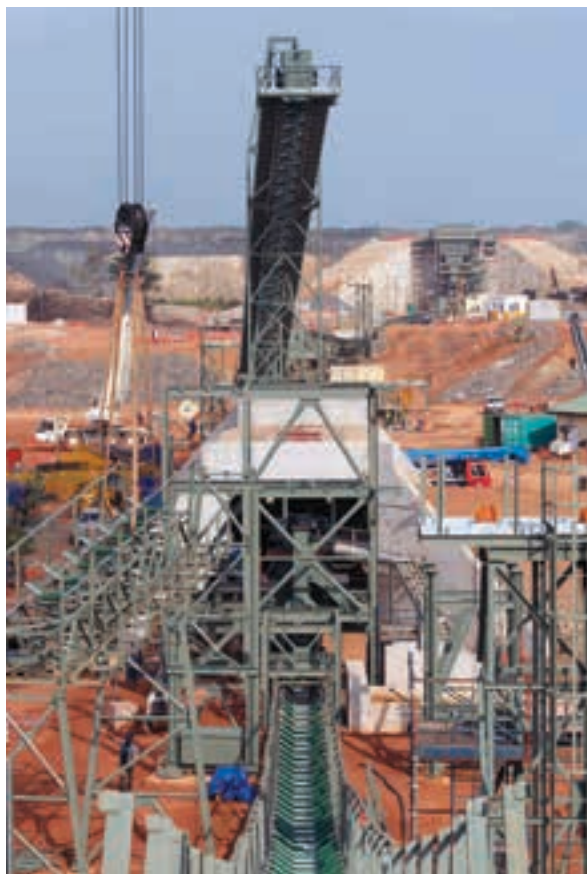
The Asanko Gold Mine site showing the stockpile tunnel (photo: Asanko Gold).
