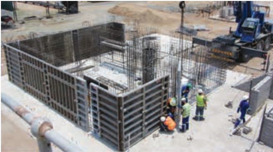
Area 300 (recovery module) at Lerala – installing QC decking in civil section of high security area of recovery (photo: Kimberley Diamonds).
