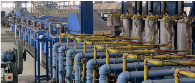
More than 75 units from QED installed
