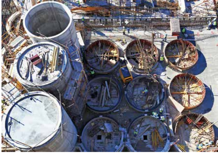
This resleeving process required concrete form work to be specifically constructed to the internal shape of the bins; this was then lowered into the bins by crane and concrete poured from the base up in a number of stages. This process was also required to form the new structure for the atrium in the centre of the building.
