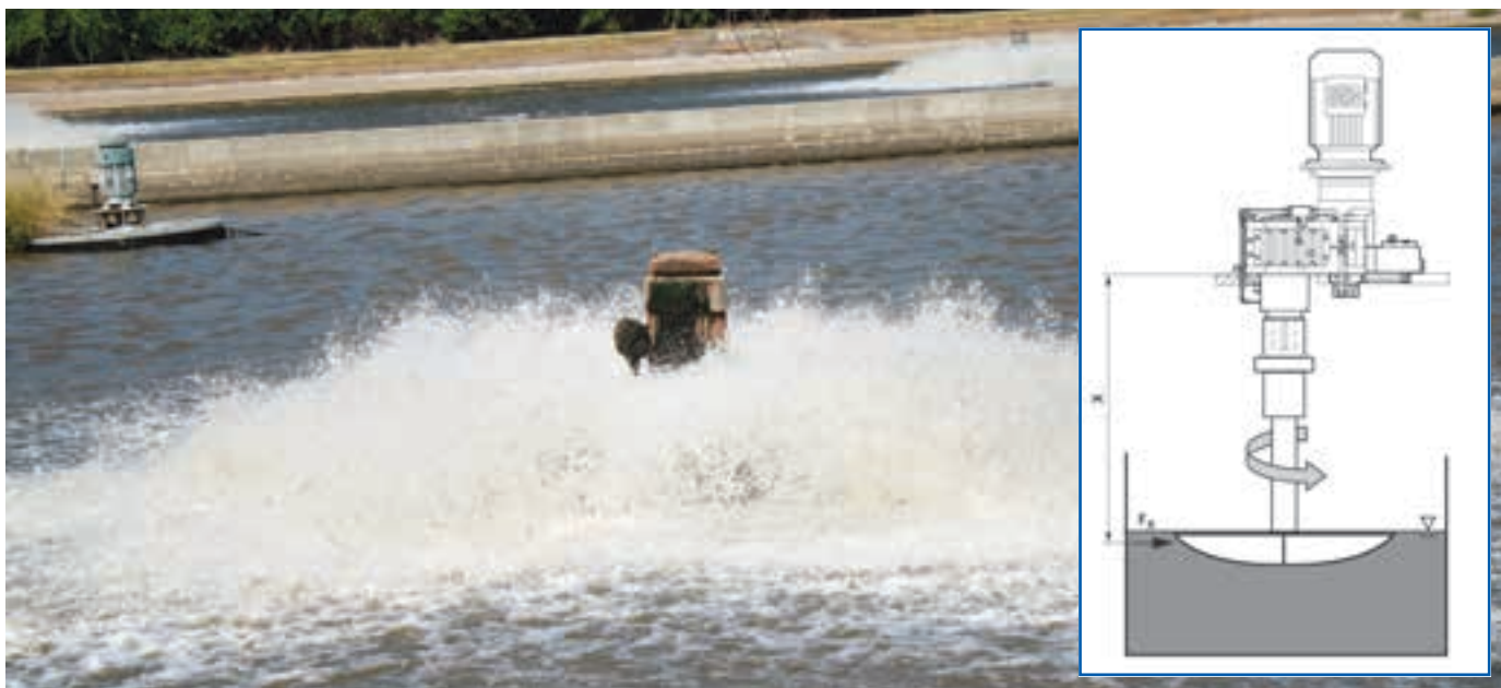
Surface aerator impeller vanes are used to pull wastewater up from the tank and discharge it horizontally outside of the impeller rim. Air and oxygen are continuously mixed, dissolved and circulated through the wastewater being treated. Inset: a layout diagram of the Meyerton aeration systems.
