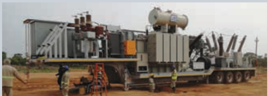
All supporting ancillary components fitted to the mobile substation. Final preparations underway, ready to commence with connection to the SNEL electrical network.
