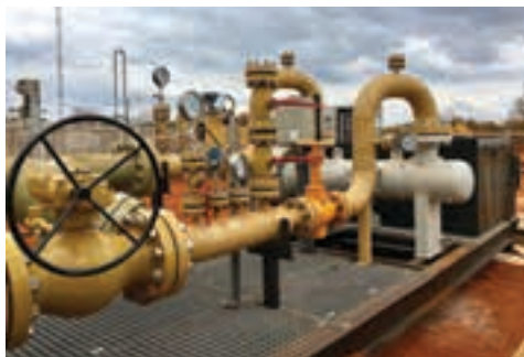
The heater skid comprises a thyristor control panel, a 416 kW heater with isolation valves, flow meter, filter, instrumentation and manually operated control valve to measure, heat and control the filling of LL2 during commissioning.
