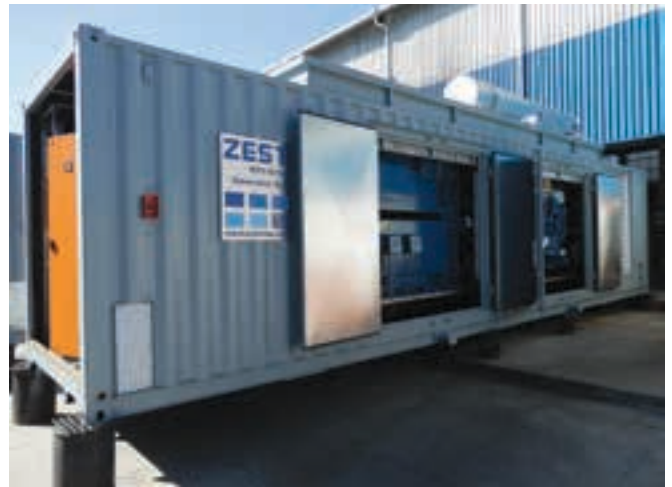
One of the diesel generator sets for Syrah Resources' Balama graphite project, custom engineered and constructed by Zest Energy.
