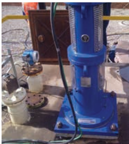
The installation of a Floway vertical turbine pump on a Multiflo barge.
