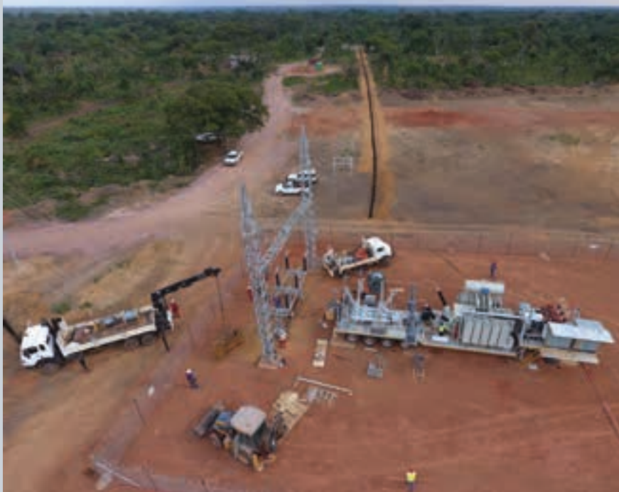
The Zest Energy mobile substation in position on site, connected to the SNEL electrical network. The photograph shows preparations for hot commissioning and energising in progress.
