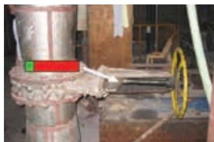
A typical gate valve in the pulp and paper industry, clearly showing the valve is approximately 90% closed.
