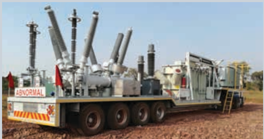
Preparations underway to start with the scope of work on site, showing the arrival of supporting ancillary components to be installed, followed by cold and hot commissioning in the presence of specialists from the DRC Utility, SNEL.
