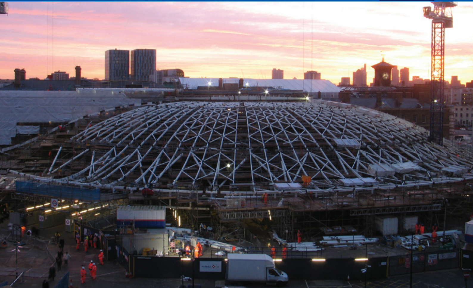
▲ Modular Wiring Systems – helping to upgrade King's Cross Station's power and lighting system
