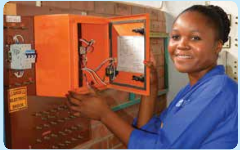
Veronica Ramashala, Level 3 electrical infrastructure learners at Tshwane North TVET College during a practical lecture demonstrating the WG MDWH miniature circuit breaker.
