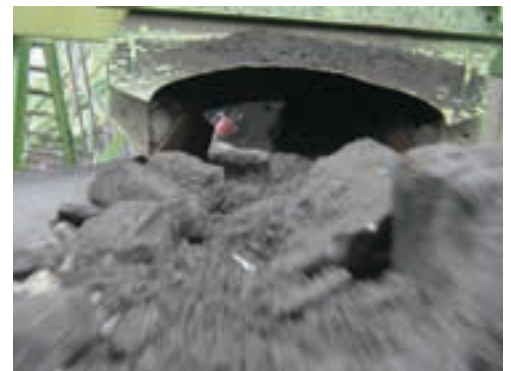
Controlling the transfer of material onto the conveyor belt guarantees increased cost savings for clients in addition to an improved health and safety performance.
