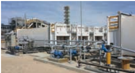
The fuel storage and dispensing facility at Husab.
