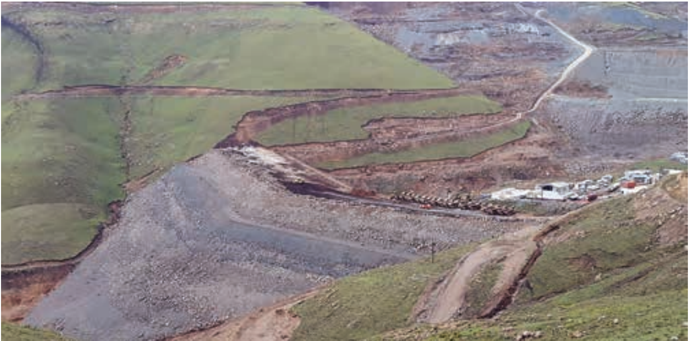
A recent view of the Residue Storage Facility (RSF). This has involved 103 000 m 3 of cut and 1,5 million m 3 of fill.
