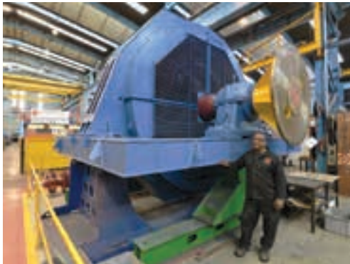
Marthinusen & Coutts's test technician, Suresh Gunpat, with the 40-pole synchronous mill motor during the series of tests conducted on it on completion of the rehabilitation process.
