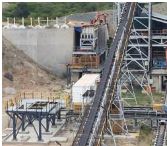
The new platform for the primary scrubber (left foreground) ready to accept the scrubber shell, the primary crusher (rear) and the refurbished conveyor (photo: Kimberley Diamonds)
