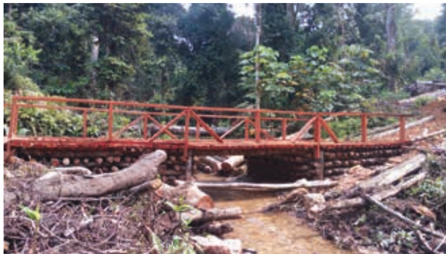
Alphamin is in the process of clearing a route from the mine site to the closest road which is about 35 km away. Seen here is a completed bridge on the route. To maximise the impact on the local economy, Alphamin is constructing the road by hand. Once the road is complete, it will allow light vehicle access to the site and facilitate construction of the final access road (photo: Alphamin).
