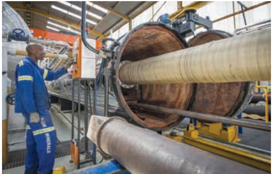
One of three autoclaves at Weir Minerals Africa's Alrode plant used to cure rubber hoses as part of the manufacturing process.
