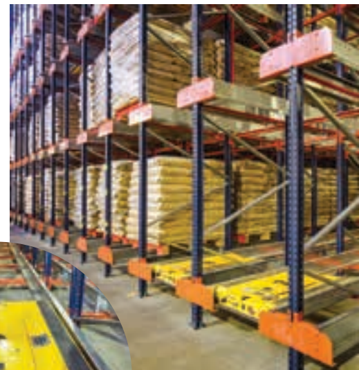
Above: The warehouse handles approximately 5 500 pallets, with total warehouse turnaround achieved fortnightly. Left: The pallet shuttle conveys pallets up to 1 500 kg at 1.3 m/s to designated storage bays within the racking lanes.
