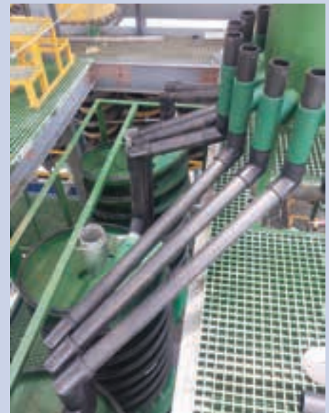
The retrofit installation of Multotec HX3 spiral bank used a custom-designed frame to suit the existing spiral building structure.
