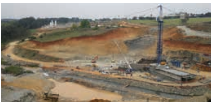
AfriSam has supplied flagship projects in KZN such as the Galleria Shopping Centre, widening of the harbour mouth at the Port of Durban and the Spring Grove Dam (picture).
