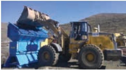
Pilot Crushtec International's Pilot Modular GFH560 is being used by EXR Construction in a Lesotho roads project.
