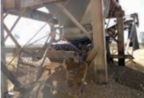
The importance of guarding, or lack of as shown in this photograph (courtesy Mr Machine Guarding, Marius van Deventer).
