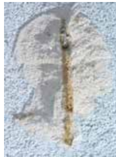
Figure 9: Unprotected aluminium down conductor – incorrect installation.
