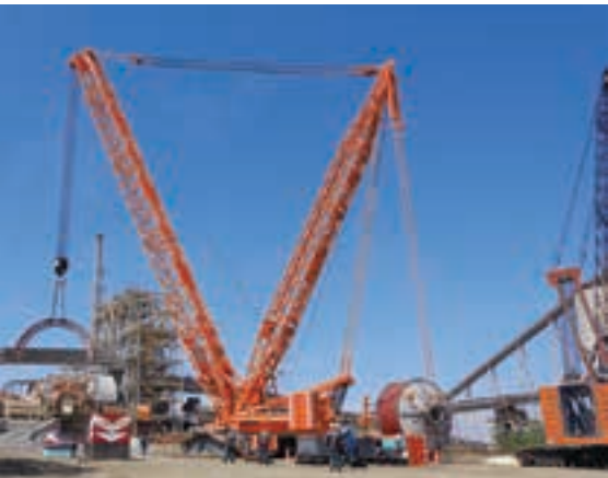
Johnson Crane Hire brought in a LR 1600/2 600 t crawler crane from Europe to take off the gears, remove the old mills and install the new one at Zimplats' Selous Metallurgical Complex in Zimbabwe for client FLSmidth.
