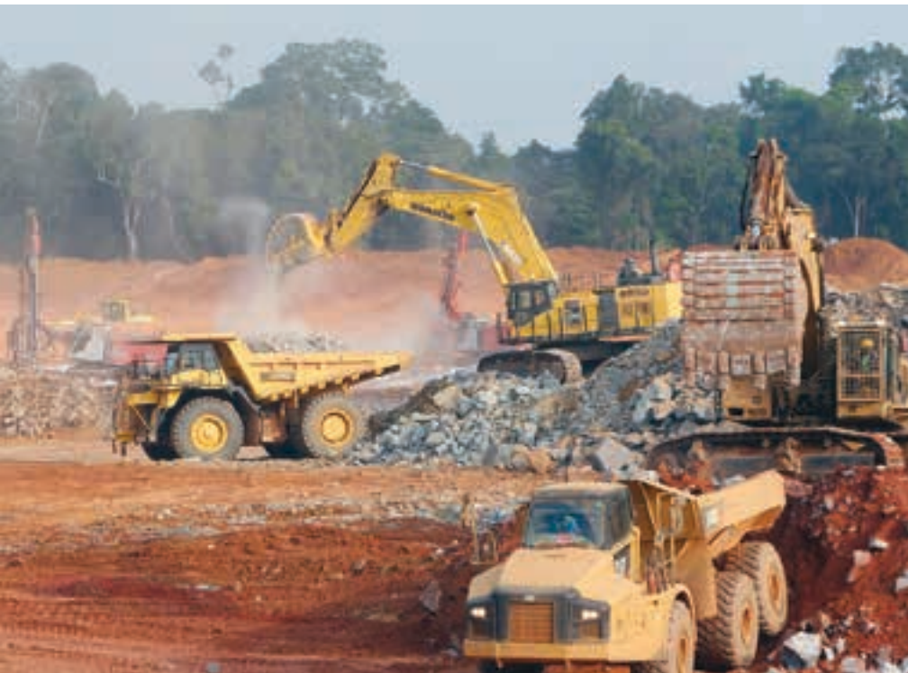
Mining equipment working in New Liberty's Larjor pit. Although Aureus is undertaking the mining itself, the mining fleet has been supplied and is being maintained by MonuRent (photo: Aureus Mining).
