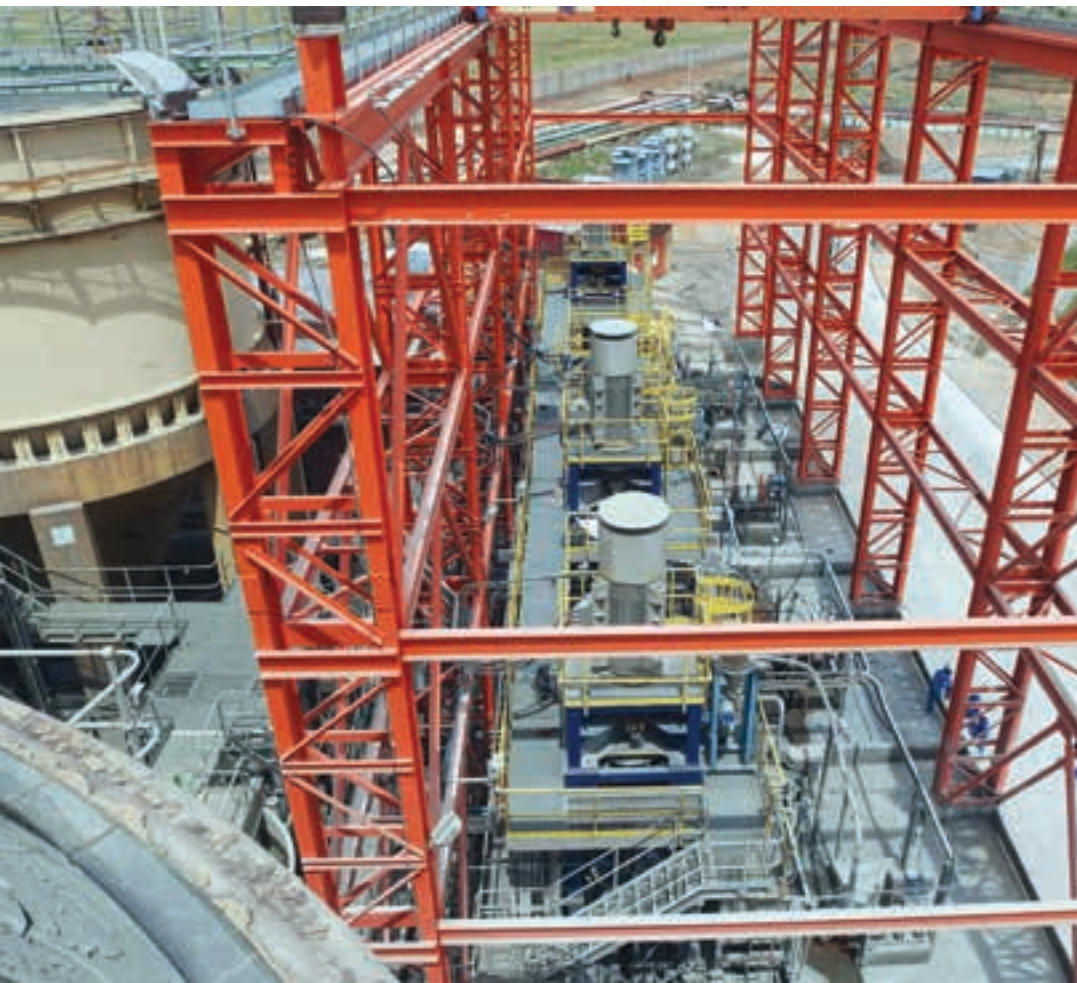
The concentrate stream is subjected to the new fine-grind process, which involves milling the slurry material with tiny beads using four vertical stirred mills, three of which are seen here (photo: Arthur Tassell).
