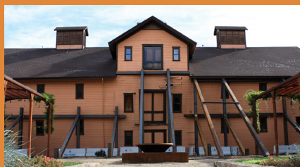
Five days later we were crushing grapes. 10 days later, a steel corset was supporting the building. Three months later, the Trefethens announced the building would be restored.
