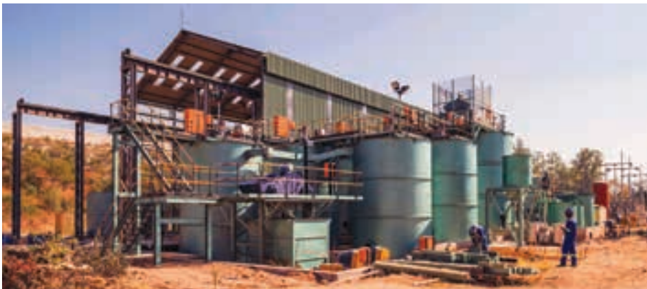
The new Mazowe processing plant as it was in early August this year (photo: Metallon).
