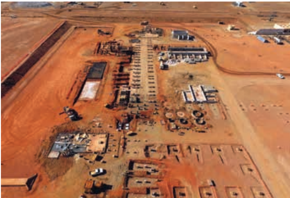
Flotation circuit plant area at Balama with concrete works underway (photo: Syrah).
