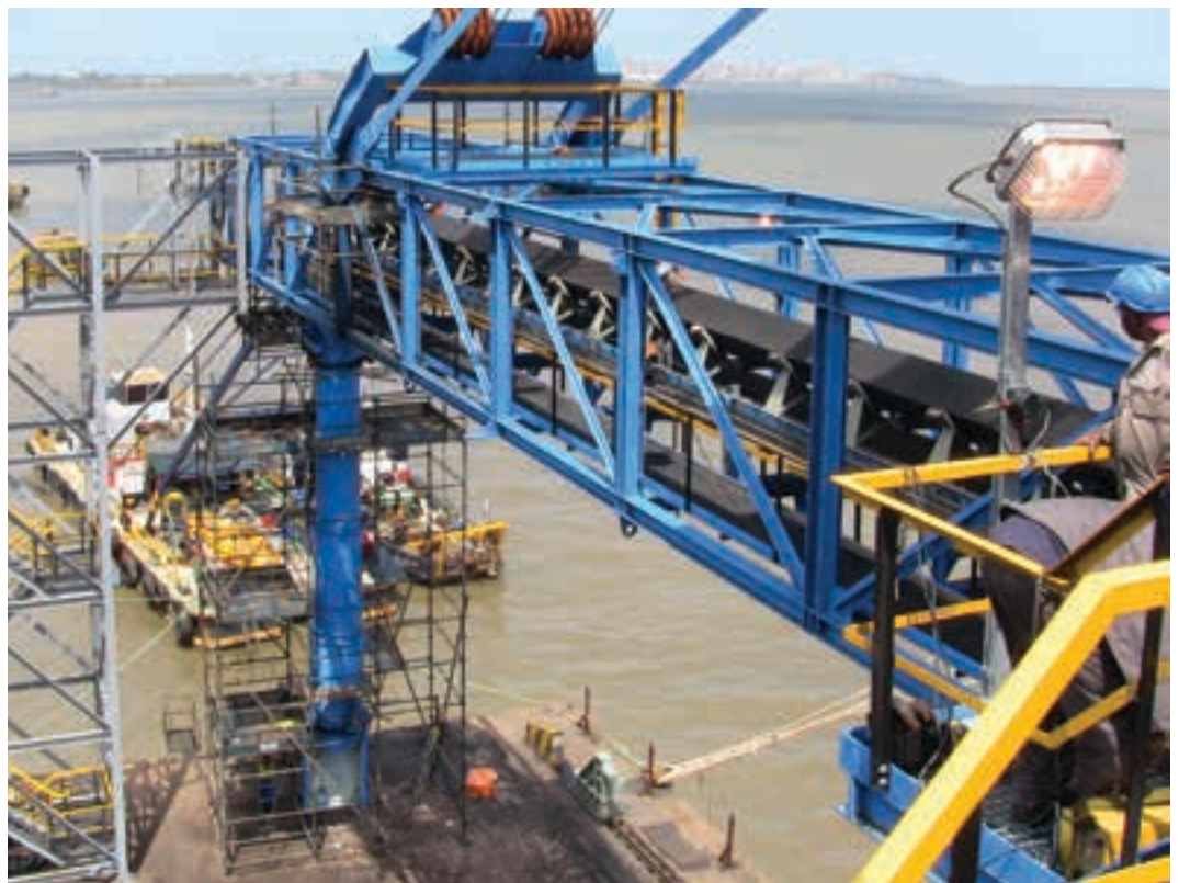
ELBCON has upgraded materials handling facilities at the Matola coal terminal in Mozambique.
