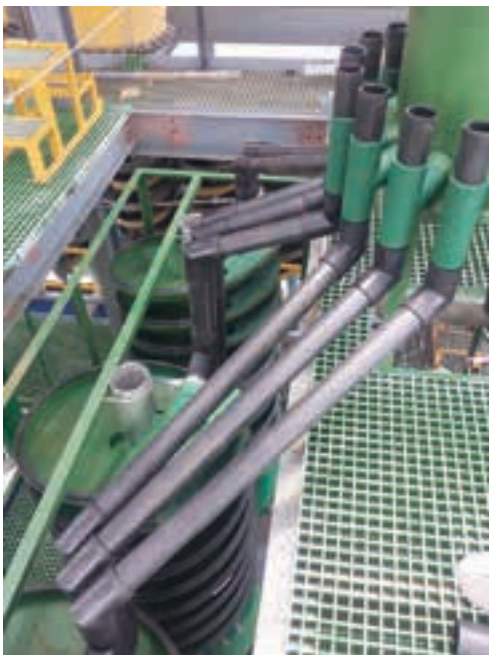
In progress retrofit installation of Multotec HX3 spiral bank in a custom designed frame to suit the existing spiral building structure.
