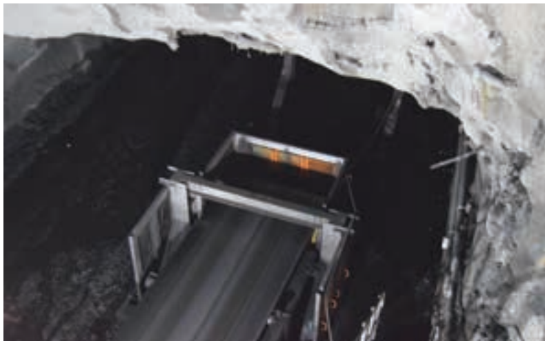
The decline conveyor seen from the box front. It has a belt width of 4,6 m/s and is rated at 2 900 tph. The extension of the conveyor under the box front was undertaken over four days in May this year.
