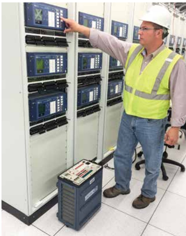
Kevin Mahoney testing the IEC-61850 based Advanced Protection and Control System (APCS) during 345 kV substation commissioning.
