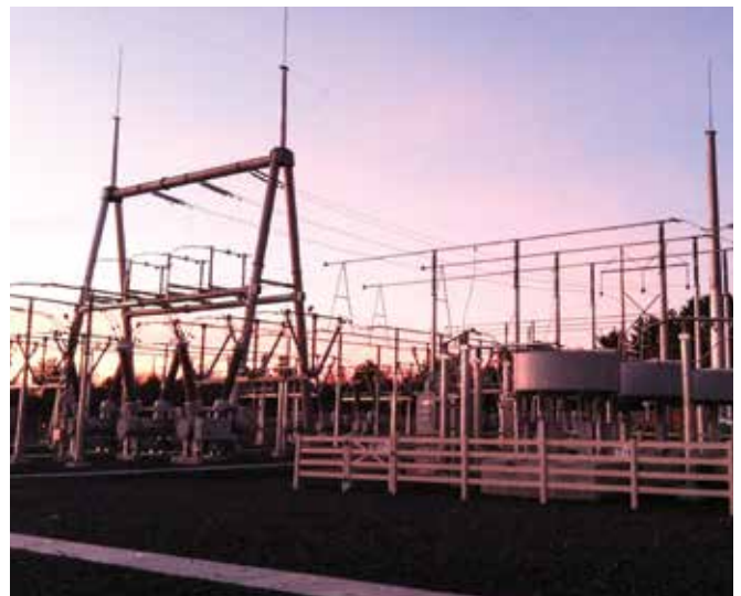
345 kV Substation Yard showing 'A' frame transmission line structure, circuit breakers and reactor bank.
