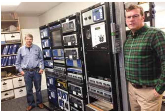
Kevin Coyne, integration engineer Casco Systems and Kevin Mahoney, founder and President of Casco Systems, with the IEC-61850 Simulation System used for Research and Development. This lab configuration was used to prototype and validate all of the integration and protection settings for the project.
