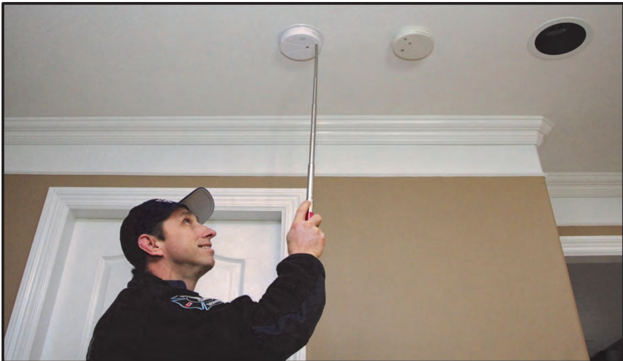
Fire crew participating in HomeSafe initiative to install and check residential smoke alarms
