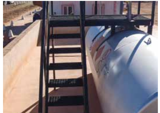
Well maintained diesel tank at IT5 Sivel Droogehout (Alan Cluett).
