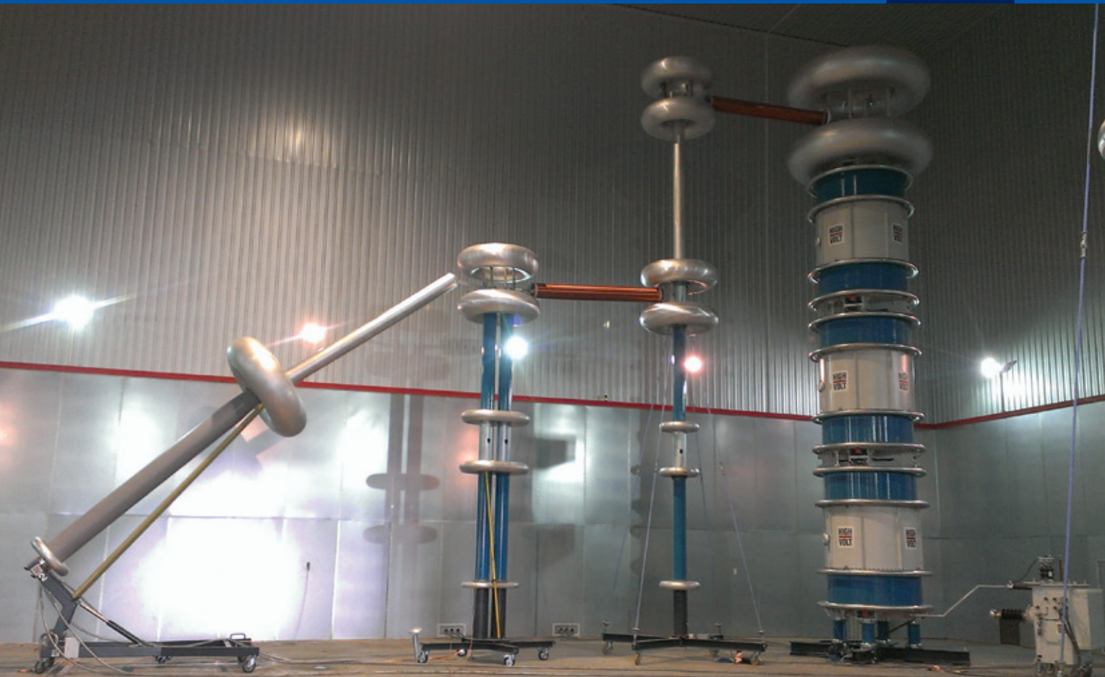
▲ Shielded cabins for testing from Highvolt Prüftechnik
