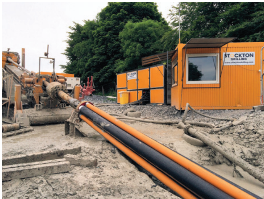
The drill rig launch site on the Galway project showing the pipe bundle successfully completed pull back
