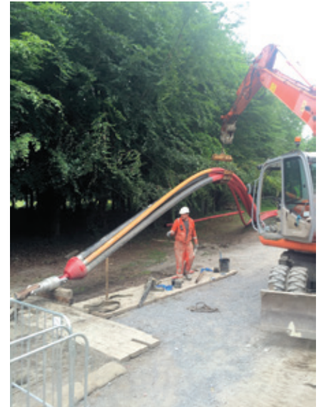
The exit side of the bore showing the pipe bundle about to be installed
