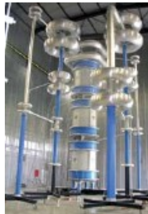
○ Highvolt AC resonant test system; photo courtesy of Demirer Kablo AS
