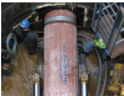
The Denlok technology in action
