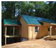
60943 - FANCY GAP - BRAND NEW HOME ON 20 ACRES, UNDER CONSTRUCTION, 2BR, 1BA, 912SF, BASEMENT, POND. $199,500
