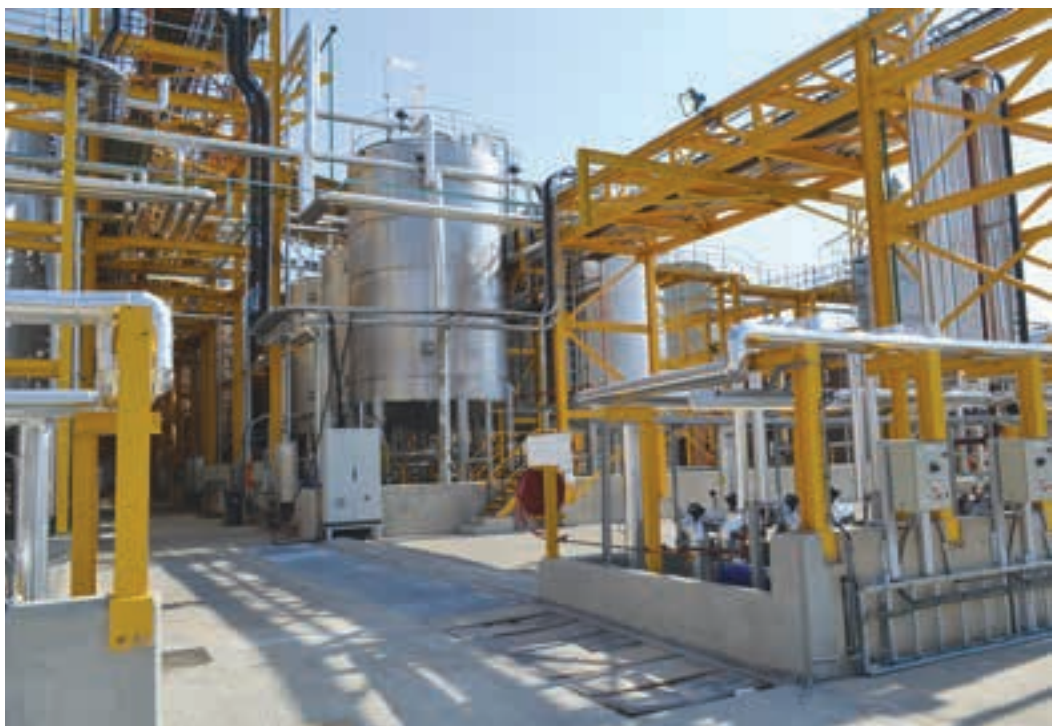
At the starting point of the Khanyisa Home Care Factory are storage tanks and a modern distribution system for the raw materials required. The factory has a capacity to manufacture 150 000 tons of liquid detergent products per year.
