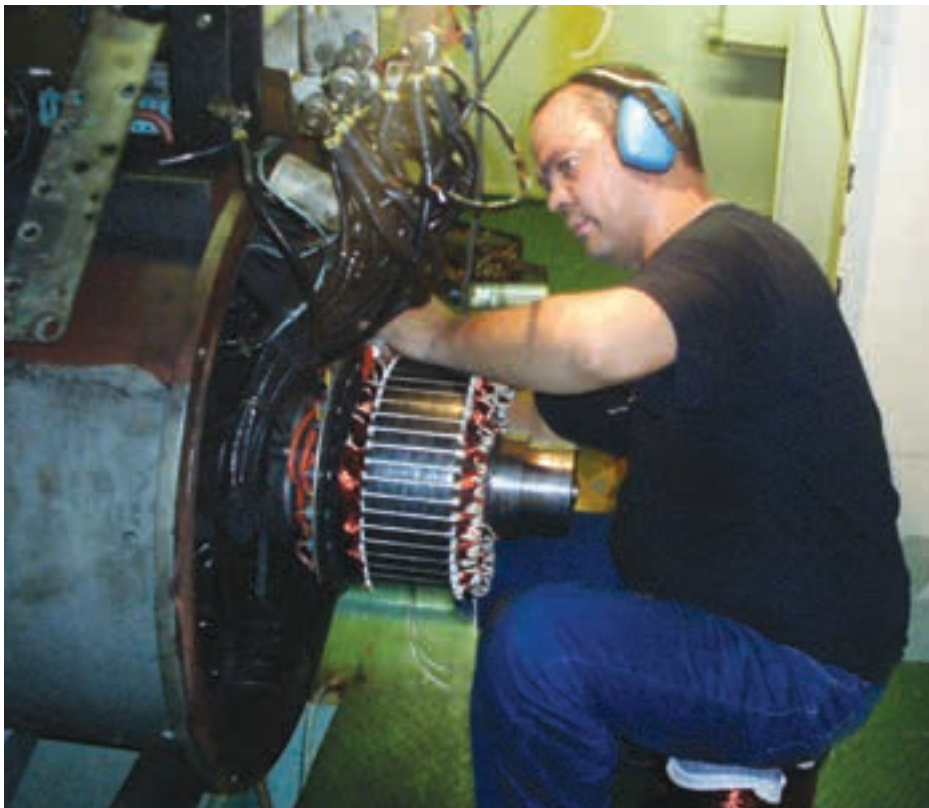
Johnny Canada, technical service manager, Vert Energy, is rewinding an exciter stator below deck on a vessel, while the vessel is fully operational.
