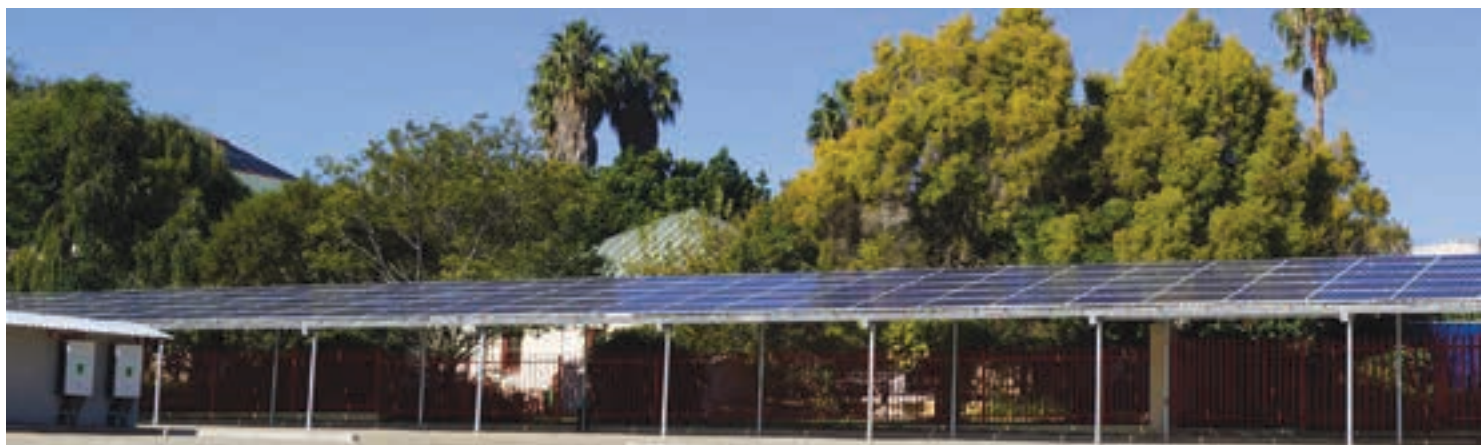
Jasco's grid-tied solar PV project at its own premises, built to proof the concept to new customers.
