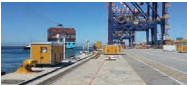
The new automated mooring units along the Ngqura quayside.
