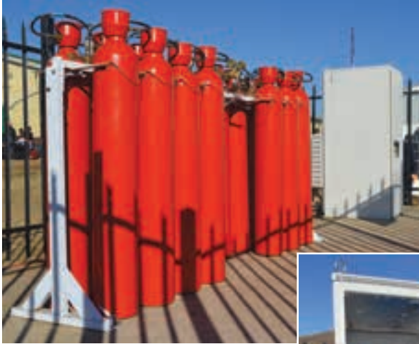
A view of the 5.0 kW hydrogen fuel cell plant at Mvuzo Junior Secondary in Cofimvaba.
