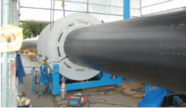
▼ Figure 2: Hot-tool butt welding is used to join the two pipe trains tension-proof with one another
