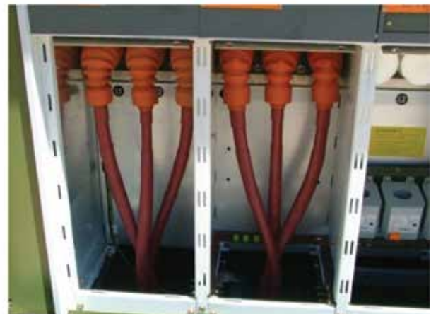
Figure 15: Example of a cable termination where the core crossing is made below the end of the core screen.
