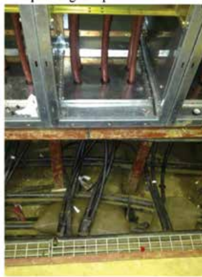
Figure 18: Example of tri-furcating termination into compact MV switchgear.
