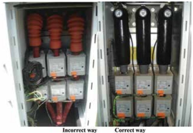
Figure 19: Example of incorrect and correct termination into compact MV switchgear with LV CTs.
