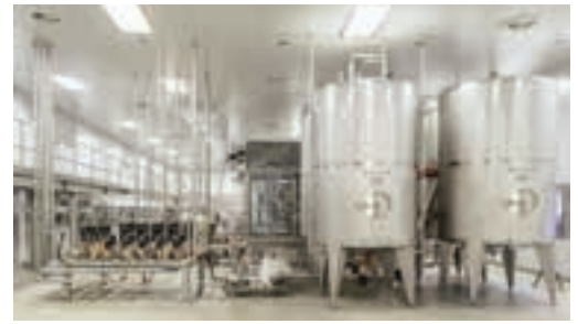
Tiger Brands' new Crosse & Blackwell mayonnaise plant in Belville, Cape Town, was installed by Stainless Steel specialist, Gerhard Unger Process Technology.
