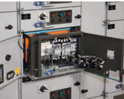
A fully withdrawable MCC board, one of the new products manufactured by Shaw Controls.
