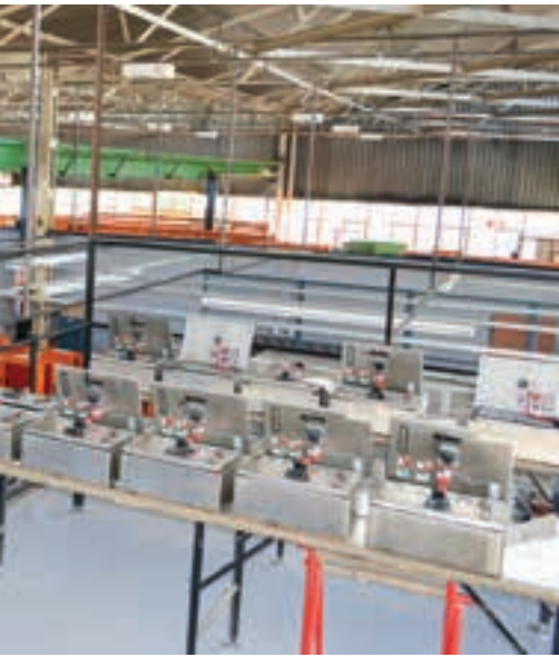
The distribution board workshop and production line at Shaw Controls.
