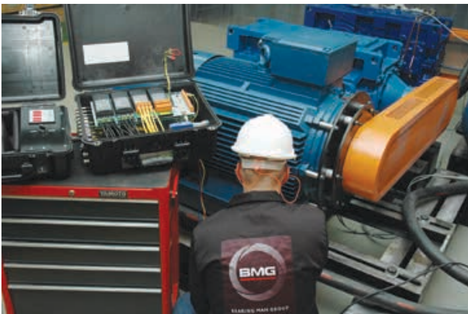
A 200 kW regenerative load test rig is being installed to support 'world class production efficiency' in South African industry.
