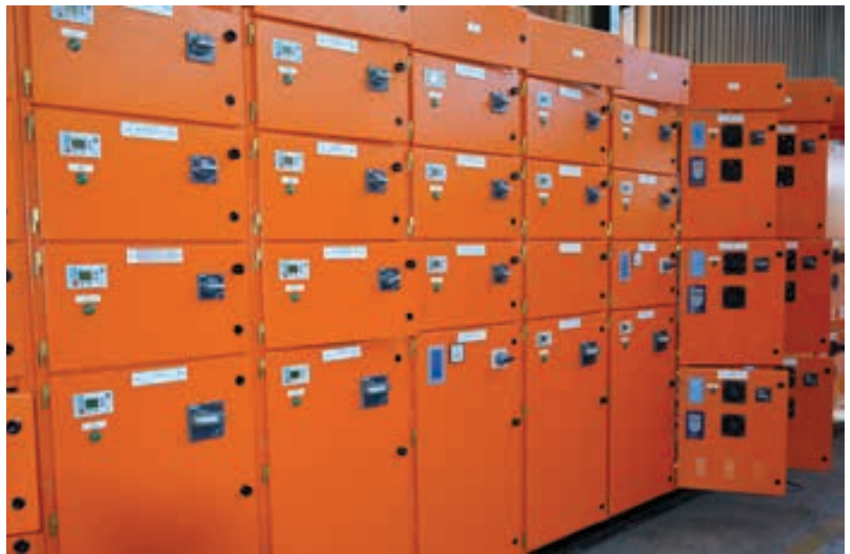
An LV fixed semi-withdrawable MCC manufactured by Shaw Controls in Robertsham.
