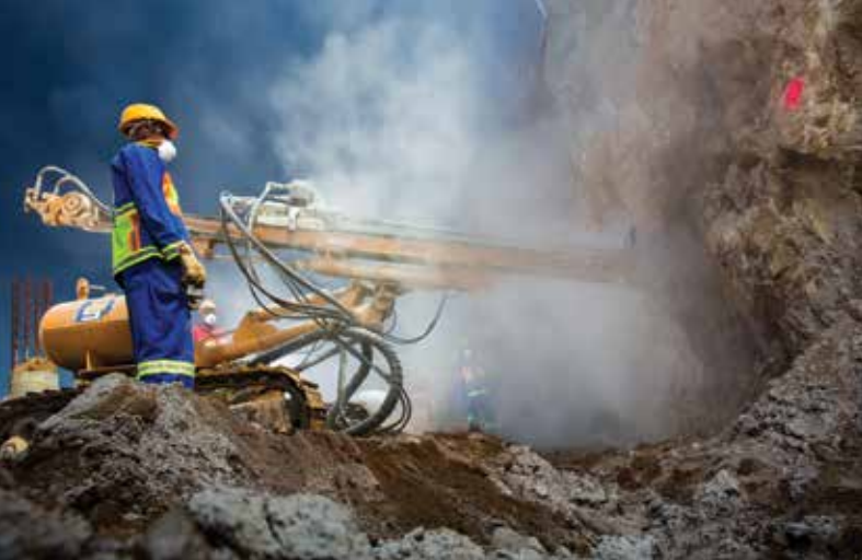
A Furukawa drill rig drilling 200 mm diameter holes for soil nail installation.
