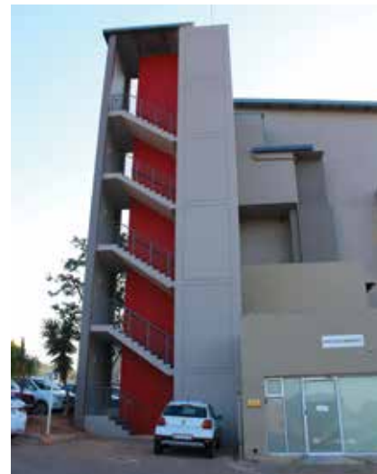
Included in the contract handled by J.C. van der Linde & Venter Projects was the installation of a new fire-escape.
