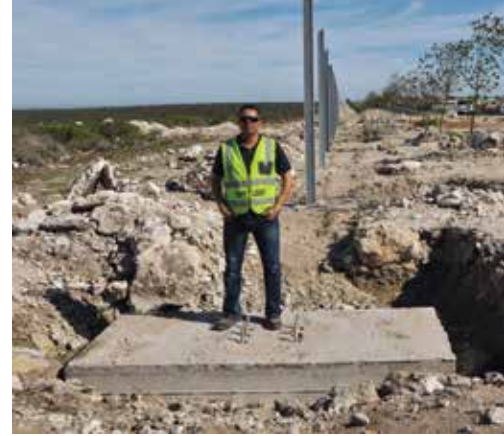
Topfloor contracts manager, Norlando Nomdoe, stands on one of the concrete foundations.
