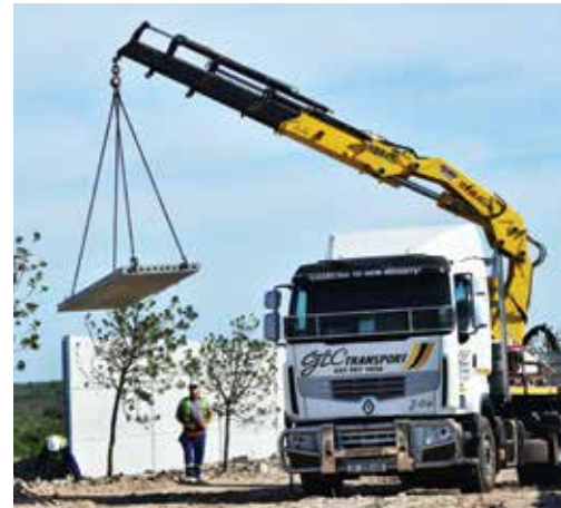
A Topfloor wall slab is offloaded prior to installation between the steel H sections.
