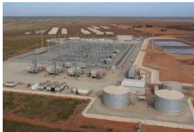
Aerial view of APR Energy's mobile gas turbine power plant in Western Australia.
