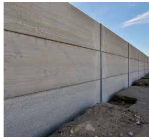
An inner section in which the attractive V-shaped indentations between the slabs are clearly visible.
