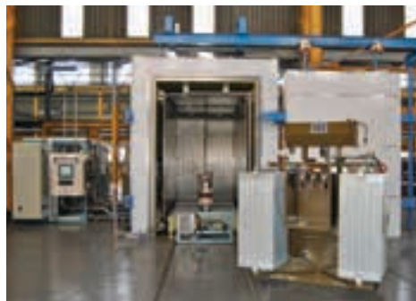
Newly Commissioned Vacuum Drying Oven
