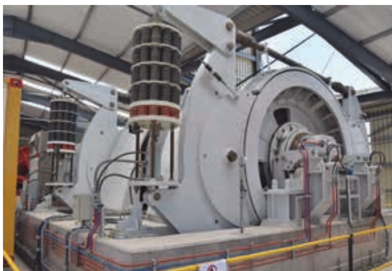
One of the winders being used in the sinking of the production shaft. The permanent winders for the project – two ground-mounted Koepe winders for the production shaft and a double-drum winder and a single-drum winder for the service shaft – have been ordered from ABB.
