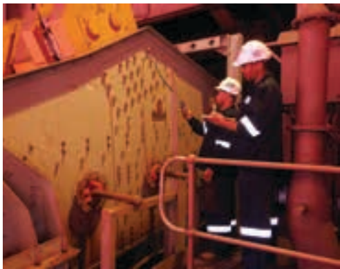
Joest Kwatani undertakes continuous audits at predetermined intervals to measure improvements in performance as well as the condition of the screen.
