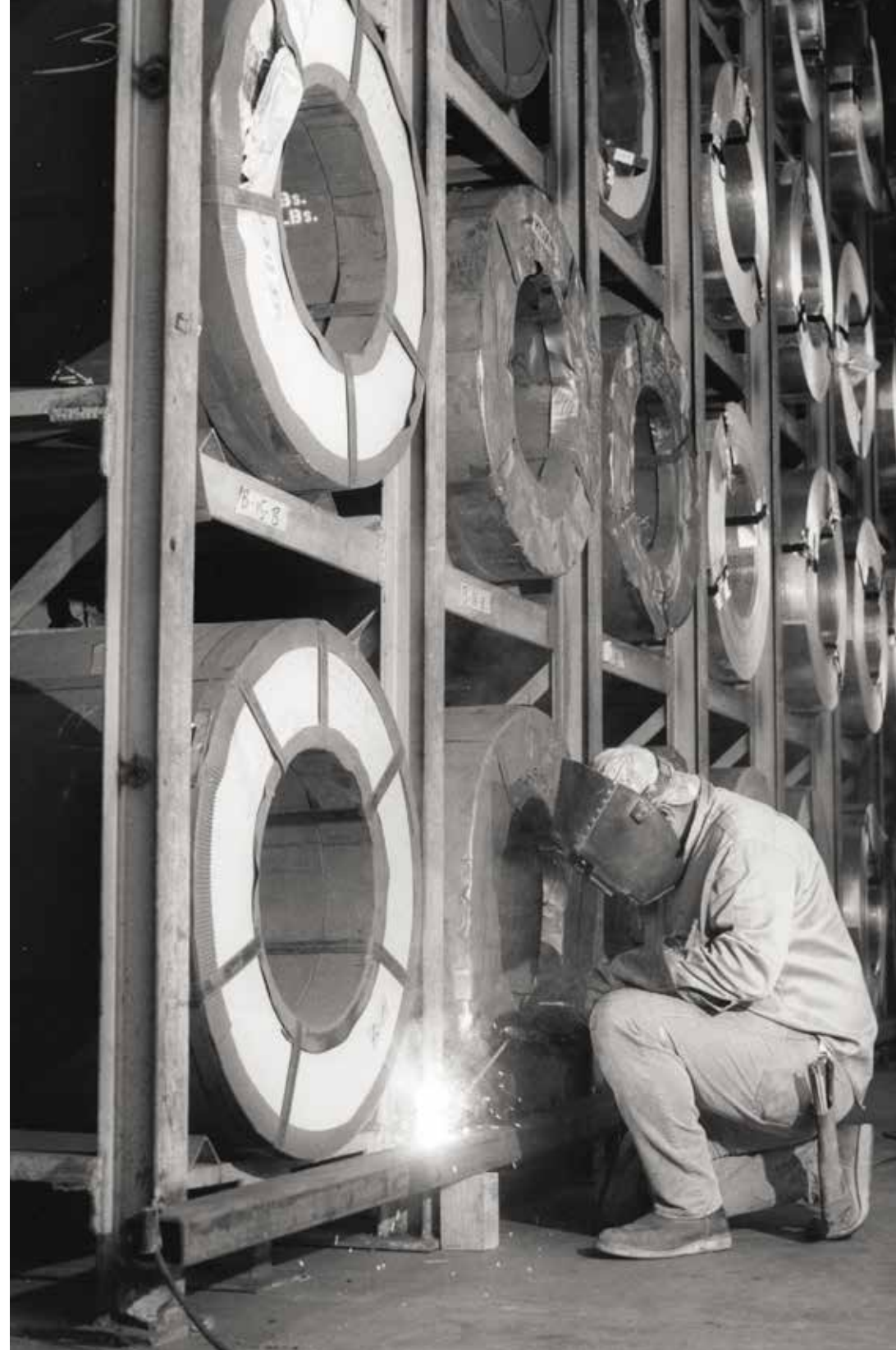
Installing a rail at the base of a five-high rack of coil, with each bay carefully numbered for efficient location and retrieval.
