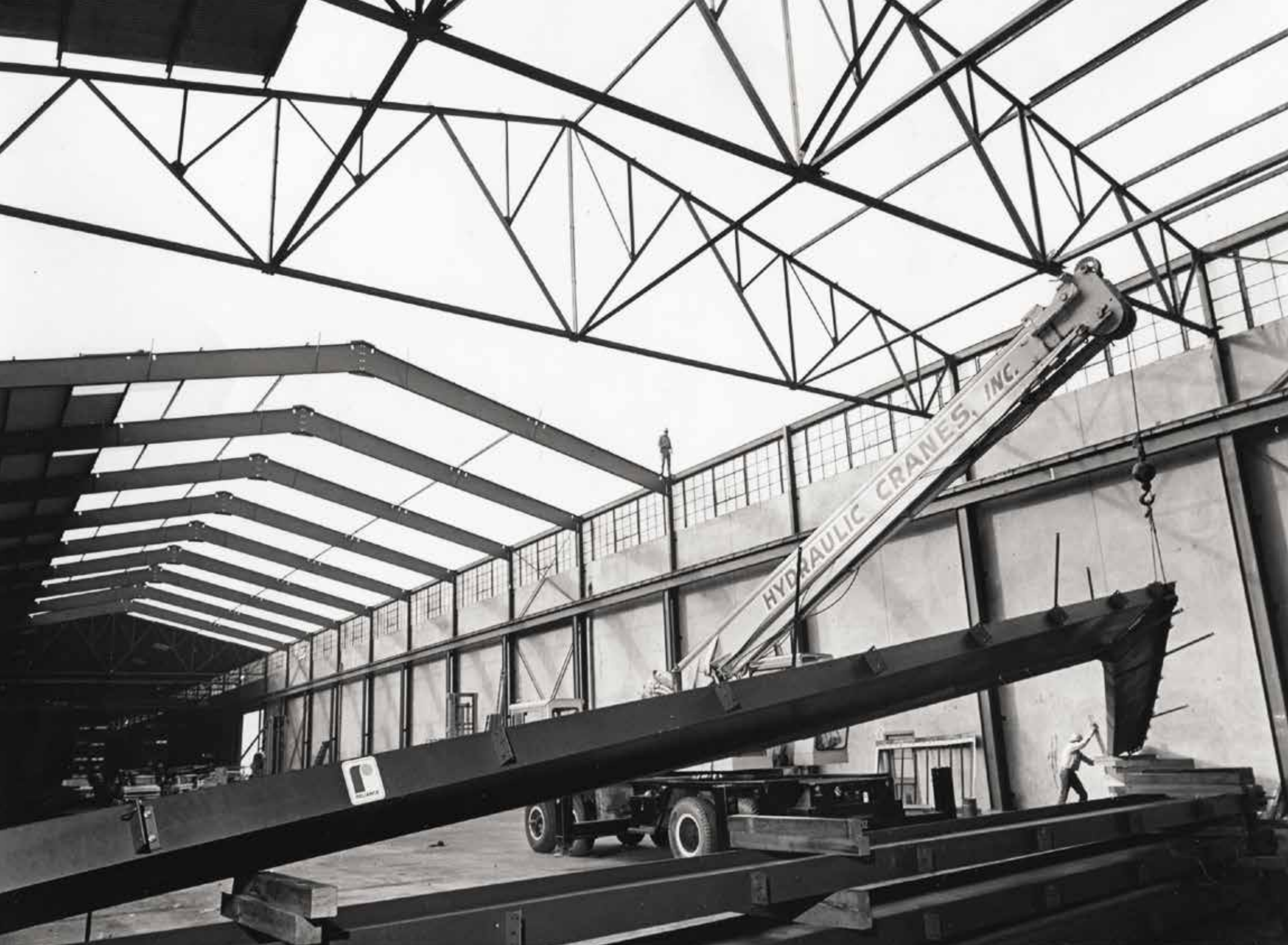
Reliance spared no effort during the 1960s to squeeze more efficiency out of its facilities. At the Vernon service center, lattice trusses (foreground) were replaced by heavy beams, thus opening up 15,000 square feet of new space.
