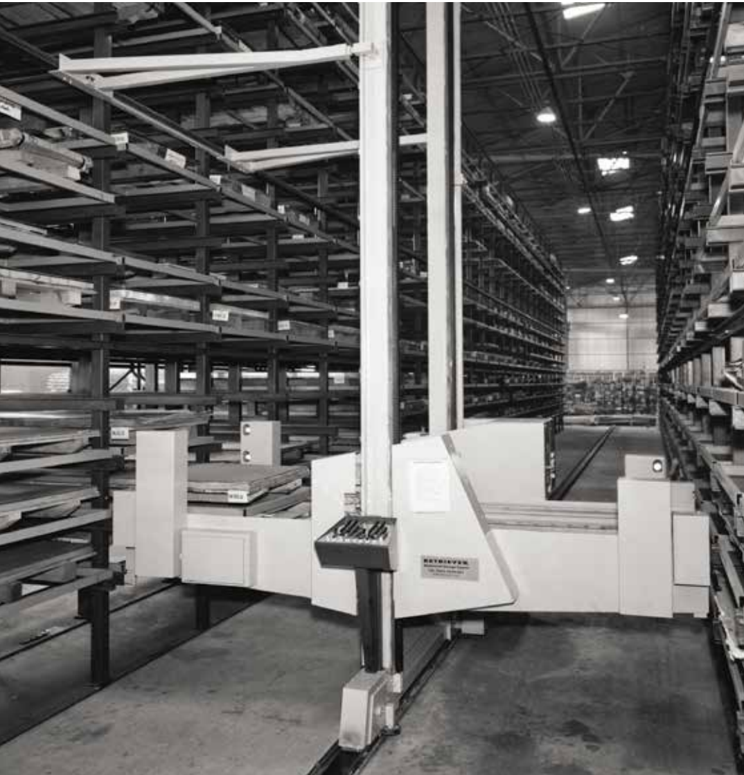
A retriever machine, part of the Triax system installed in 1962, takes sheet metal from one of 1,850 pigeonholes.
