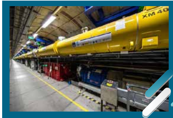
View into the 2.1-kilometre long accelerator tunnel of European XFEL with the yellow superconducting accelerator modules hanging from the ceiling (photo: DESY/D. Nölle)
