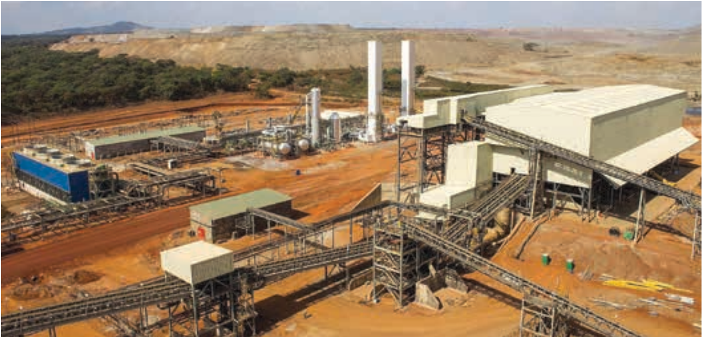
The new FQM smelter at Kansanshi in Zambia showing the smelter reagents building and the oxygen plant (photo: FQM).
