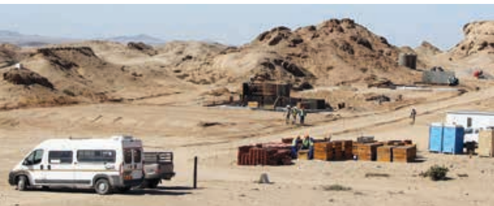
Construction activities underway at the demo plant site at Etango (photo: Bannerman Resources).
