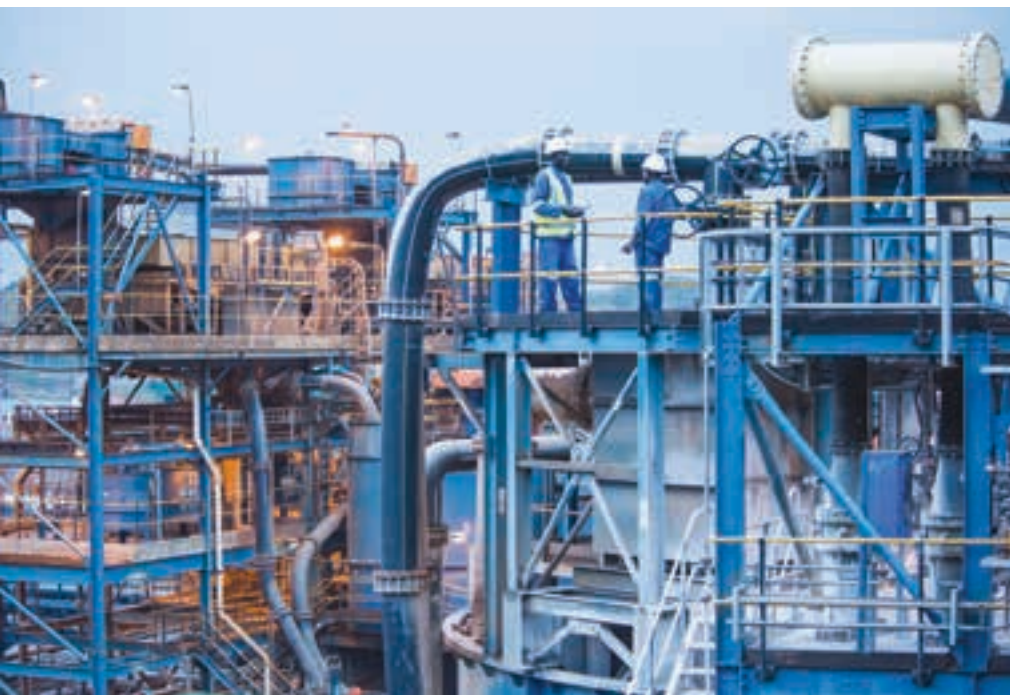
A section of the twin-circuit (oxide and sulphide treatment and sulphide only treatment) metallurgical plant at Kibali. Both circuits are designed for 3,6 Mt/a. The plant has now been fully commissioned and is meeting design parameters (photo: Randgold Resources).
