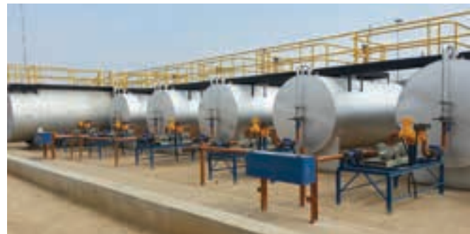
Holding tanks – of 1 000 and 20 000 litre capacity – store the various lubricants and coolants required at the North Mara gold mine site.
