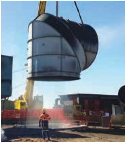
This picture shows the new shaft top being lowered into place over the mouth of Black Rock mine's 500 m deep main vent shaft.
