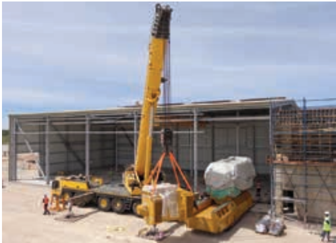
Johnson Crane Hire recently successfully completed a specialised lifting solution at the B2Gold Otjikoto project in Namibia.
