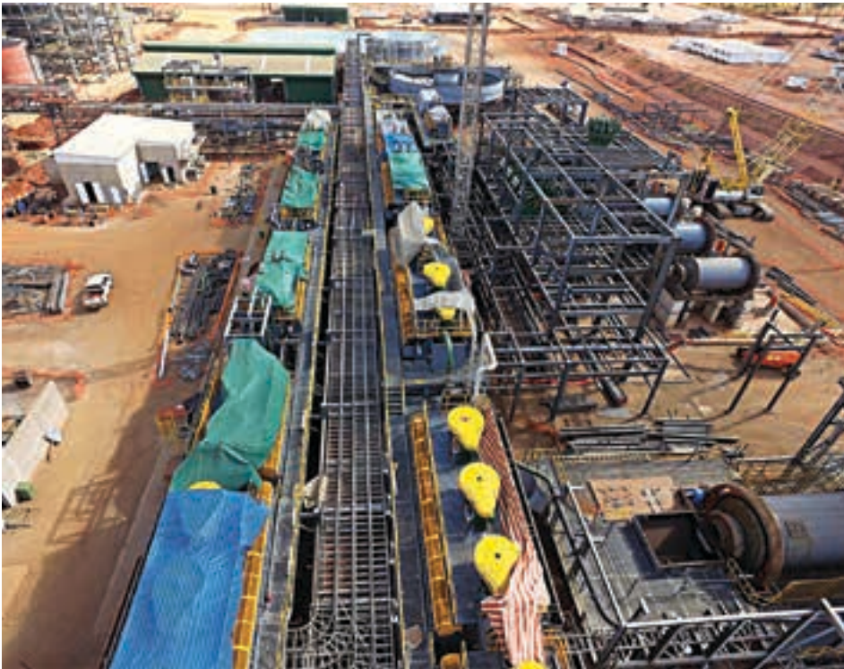
The flotation section of the Balama plant under construction (photo: Syrah Resources).
