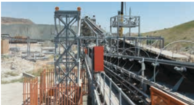
Weba Chute Systems uses three-dimensional (3D) scanning technology to ensure high quality results.
