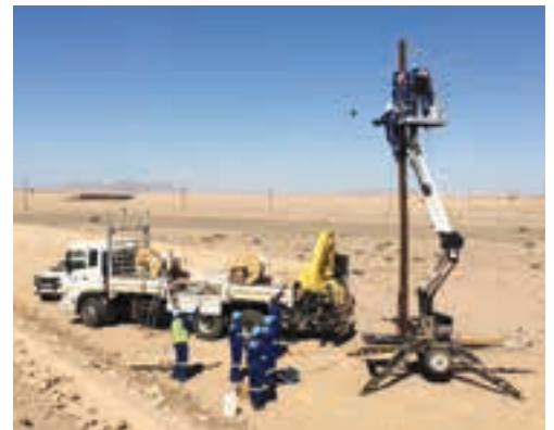
Stringing a 33 kV OHL (overhead line) at Enl Electrical's contract at Husab in Namibia.
