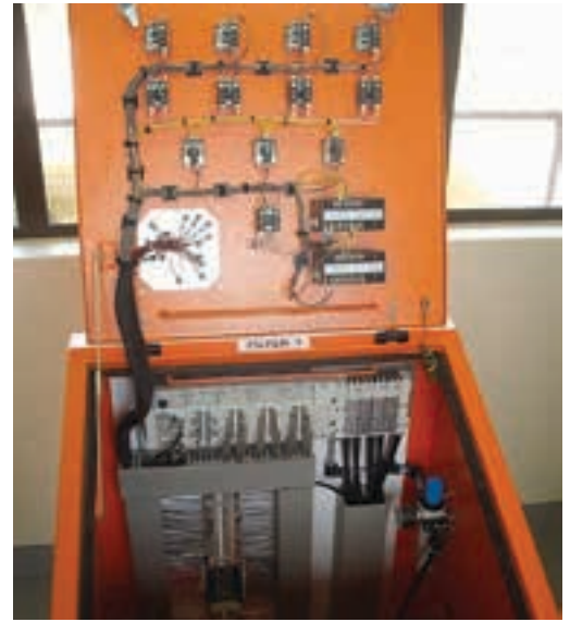
In response to the need to drain the compressed air lines regularly to prevent pneumatic actuators from absorbing damp and corroding. Festo now installs automatic dump valves on timers that will ensure that the filters are timely and adequately drained.
