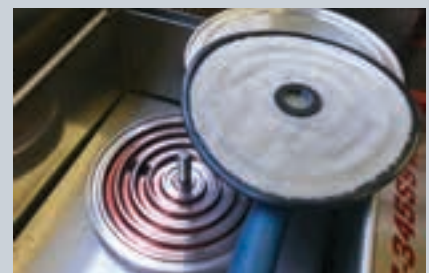
The return line passes over a 10 µm filter that enables visual checking to ensure that all debris has been cleared and the lines are completely clean. Shown here is a view of the final flush of the screen filter.
