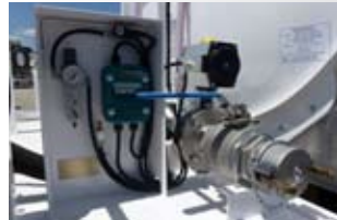
Liquip MPP102 tank monitor system for overfill protection
