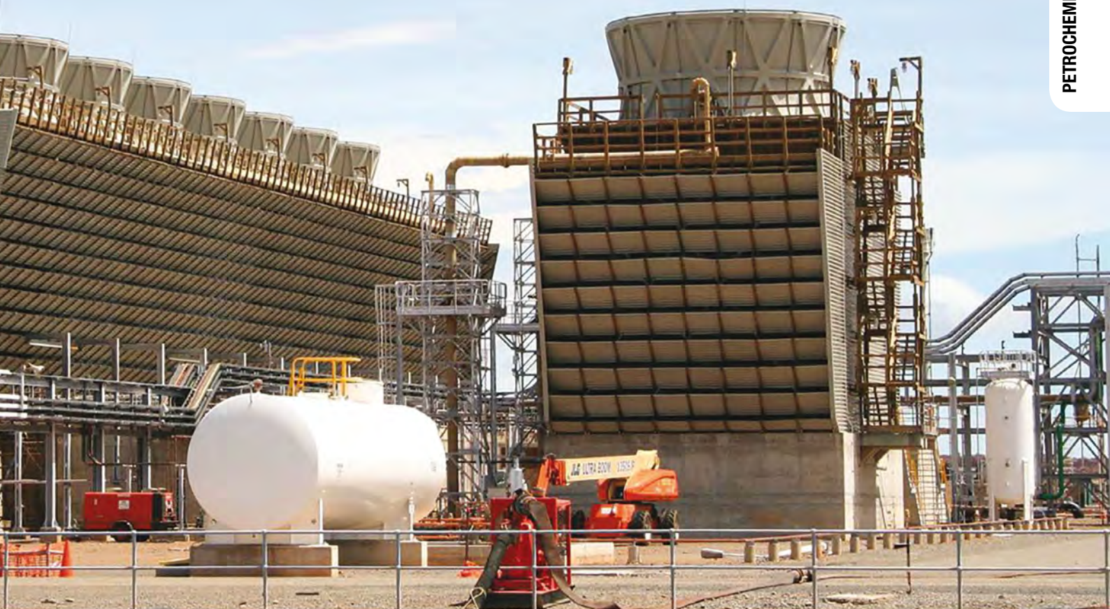
Figure 1: Cooling towers at many refineries have old instrumentation, some of it out of service.
