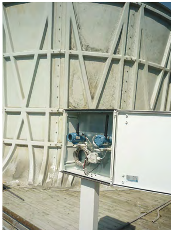
Figure 3: An enclosure protects WirelessHART transmitters from the corrosive environment near cooling towers.
