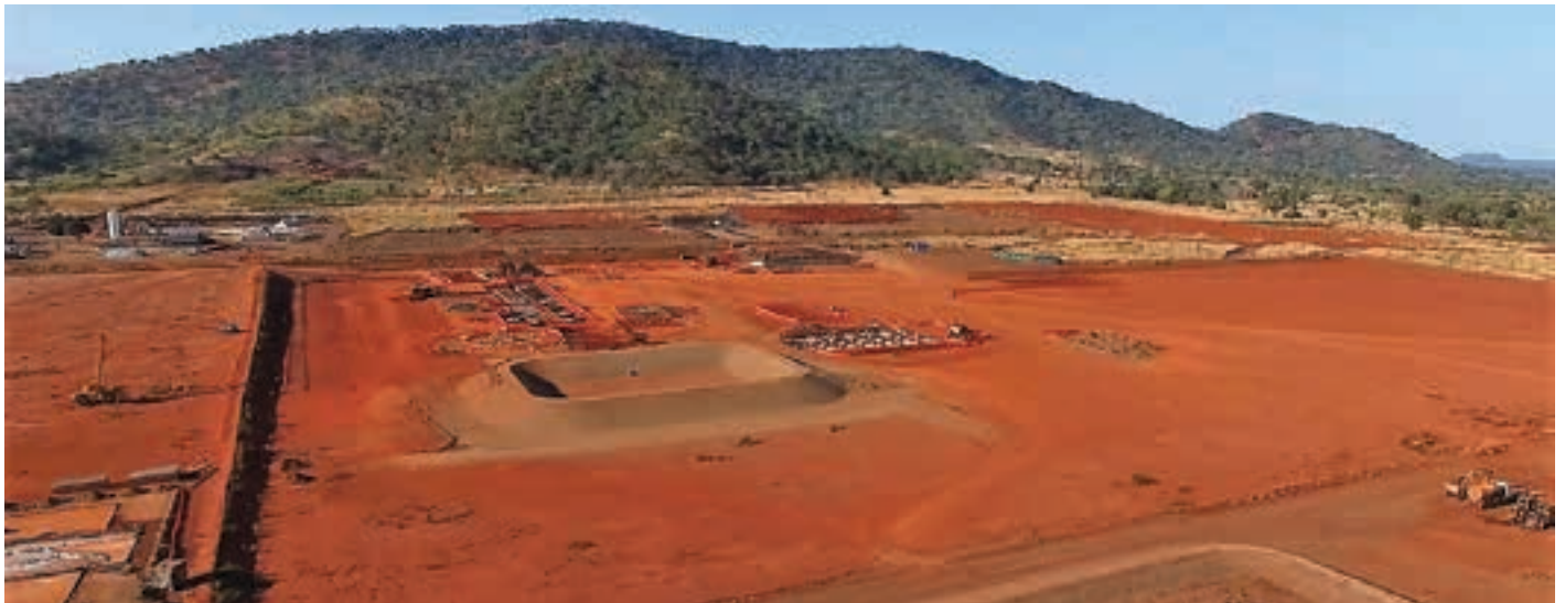
The Balama site where concrete works have commenced in the key areas of the crushing facility and primary mill foundations (photo: Syrah Resources).
