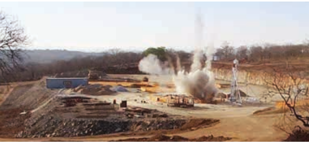
First blast at the Central Shaft in September 2015. The 6 m diameter shaft is being sunk to a depth of 1 080 m and will have a hoisting capacity of 3 000 t/day (photo: Caledonia Mining).
