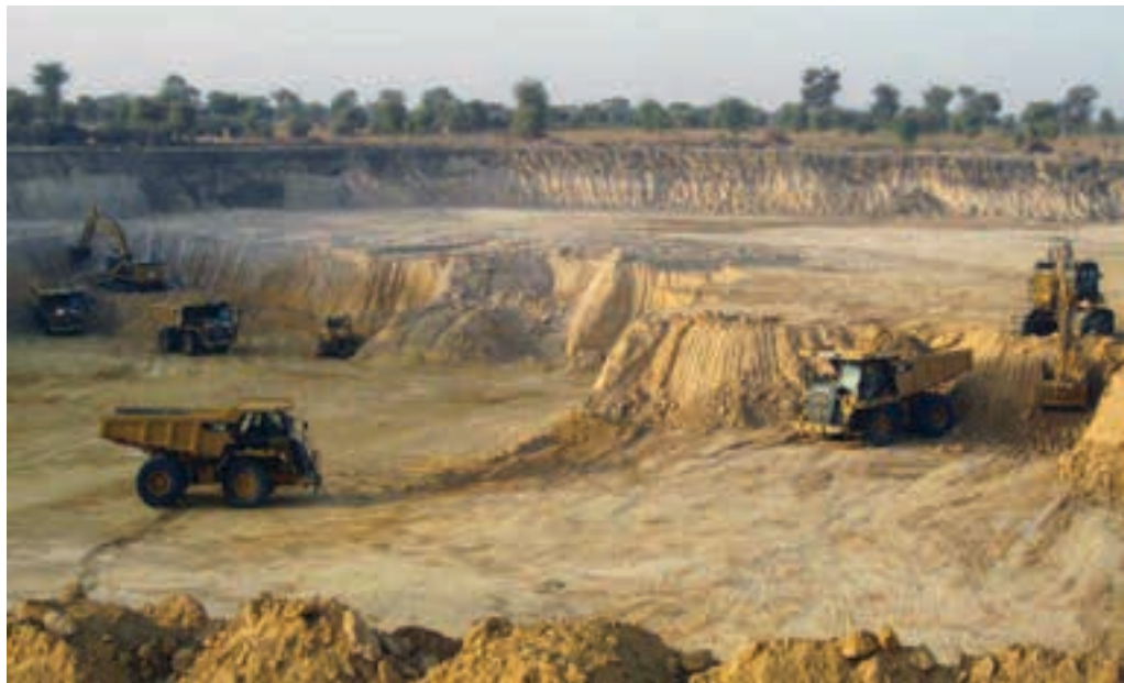
Overburden removal at the Baobab site by mining contractor Agromines (photo: Avenira).
