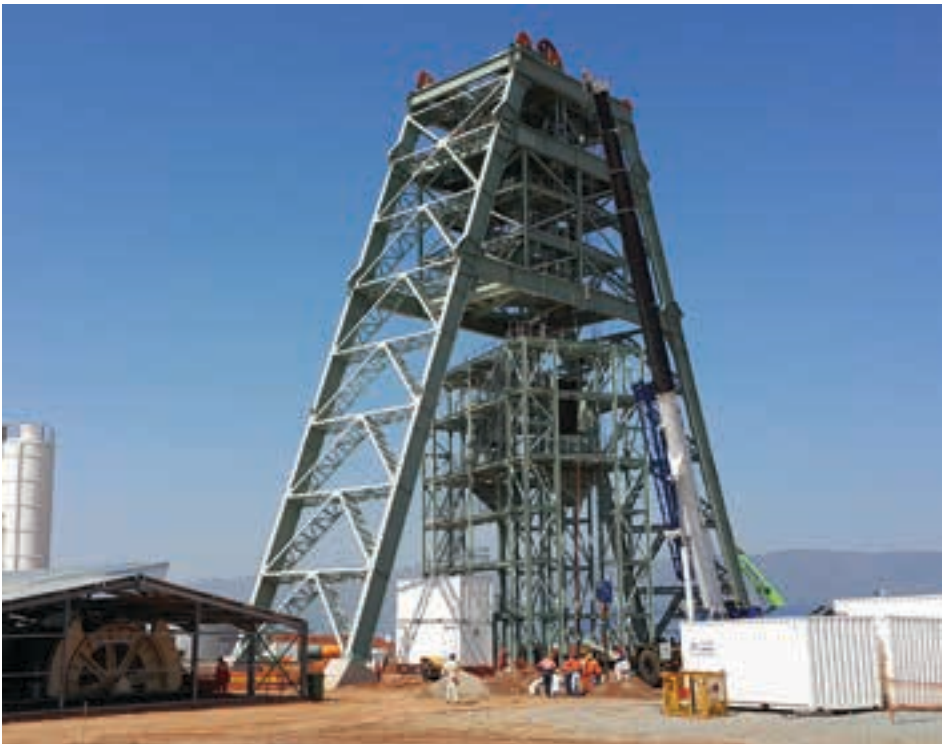
The Platreef site near Mokopane showing the Shaft 1 headgear (photo: Arthur Tassell).
