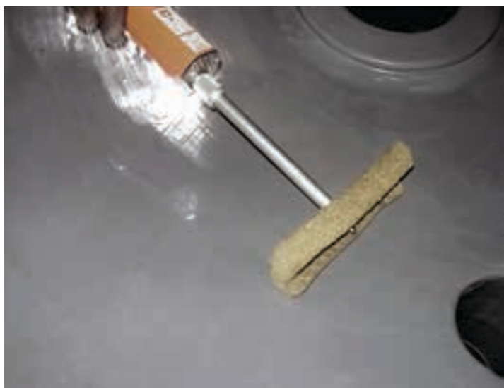
Figure 3: A paste grade epoxy material was chosen to fill the pits and afterwards, the wall was protected with a modified epoxy novolac coating.
