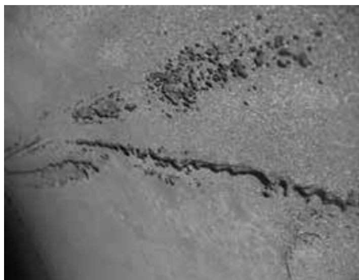
Figure 2: An amine reboiler vessel at a UK gas terminal was discovered to have suffered heavy pitting corrosion.
