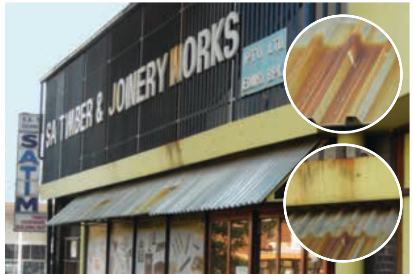
In Johannesburg, where uncoated zinc roofs are positioned below steel railings, security barriers or similar – typically on roofs built over pavements outside shops – the dissolved rust runs off from the upper level, rapidly rusting the sheeting below.
