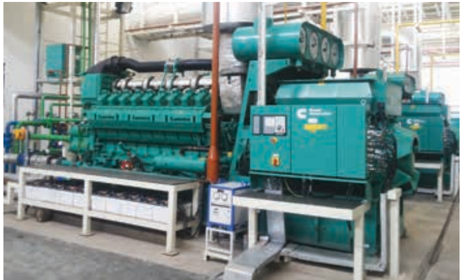
Cummins’ natural gas-fuelled QSV 91 generator sets are ideal for CHP (combined heat and power) applications such as data centres, where cooling dominates the load profile: this because the exhaust gas stream runs significantly hotter – by about 200 °C – than diesel-engine equivalents.
