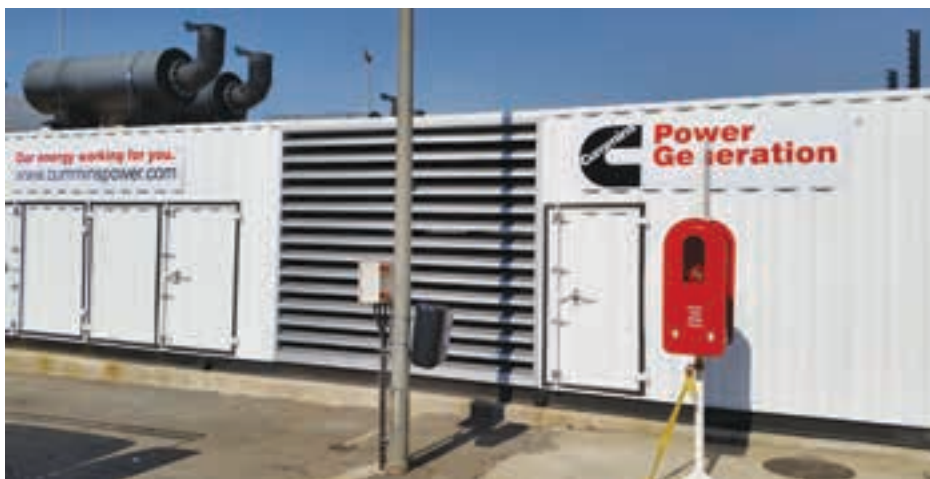
The SABMiller Polokwane Brewery in Limpopo was supplied with two fully containerised C1675 D5 gensets with a prime rating of 1 400 kVA each.
