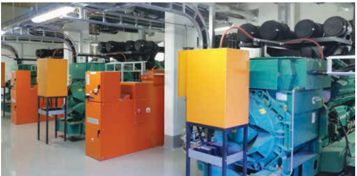
Cummins supplied SABMiller Alrode Brewery with four C2500 D5A diesel generator sets for emergency standby power. The 6.6 kV generators boast a prime rating of 1 800 kVA, and are powered by a Cummins QSK60G8 engines.
