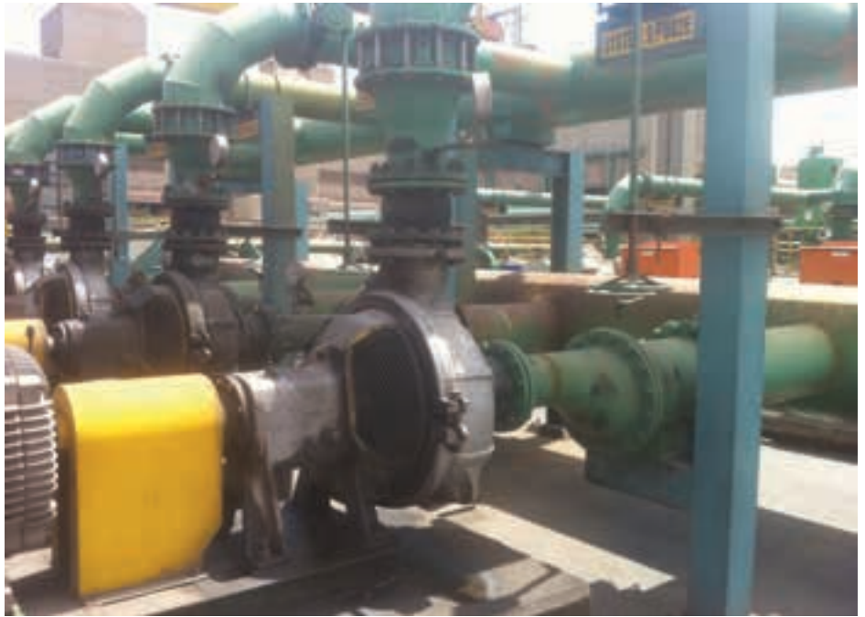
Figure 2: Pumps in parallel often have their discharge valves throttled to ensure that the current drawn is kept below the maximum motor rating. The author has found numerous instance where the current drawn is far less than maximum motor rating and fully open valves do not overload the pump motors.
