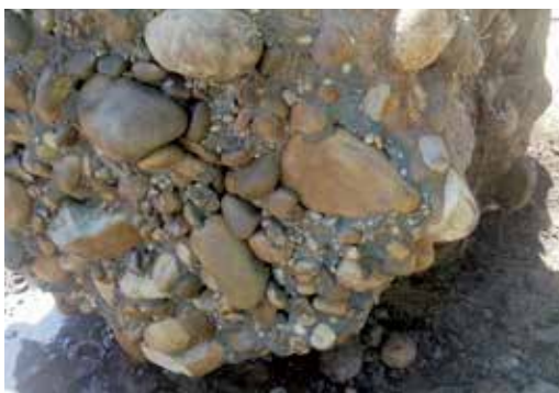
BELOW: Exposed trial jet grout column clearly showing dense cobbles that are bound together after treatment.
