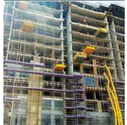
Bricks are lowered by crane onto a landing on the south-facing side of the building.
