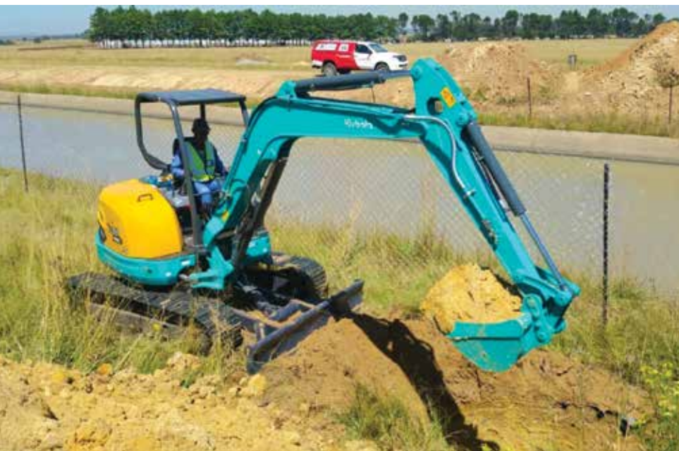
Pipe Jack Gauteng's Kubota U50 compact excavator at work on the pipe cracking and pipe laying contract for Rand Water Board.
