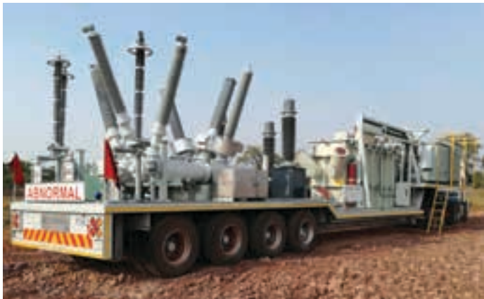
The mobile substation in position on site, with supporting ancillary components still to be installed.
