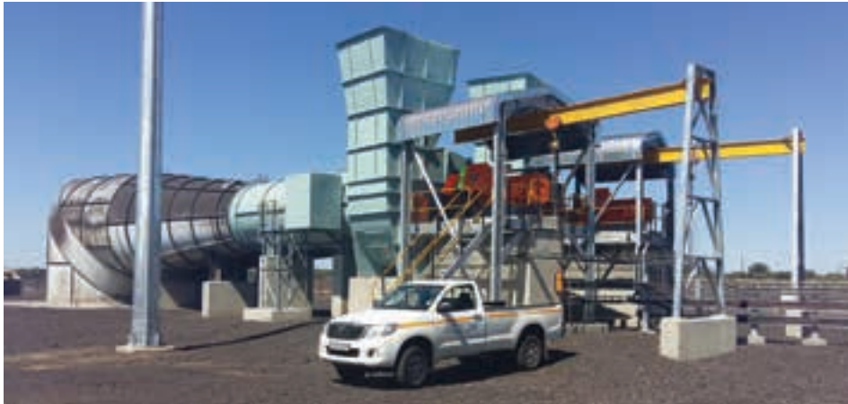
The main ventilation fan system at Black Rock Mine Operations' Gloria ventilation shaft.
