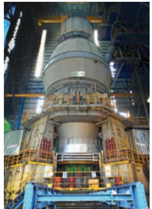
The LM 70.4+4 CS mill in operation with the new COPE drive at the cement plant in Mfamosing.
