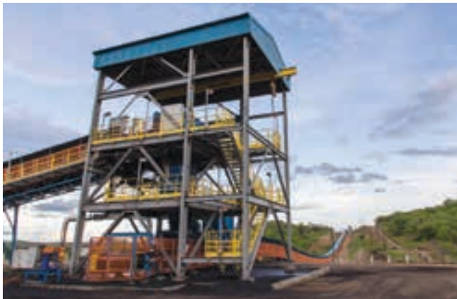
A typical conveyor transfer point. FLSmidth Roymec uses a sophisticated proprietary software program which facilitates absolute control of all elements of the conveyor build.
