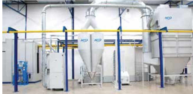
The green pre-treatment facility.
