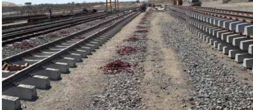
Chryso SA supplied the admixtures and demoulding oil for the production of concrete railway sleepers for Mozambique's Tete to Ncala railway line
