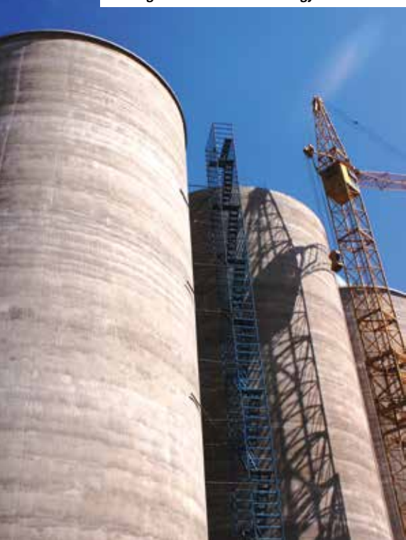
Construction of six grain and wheat silos in Kimberley in the Northern Cape using slip forming construction methodology.
