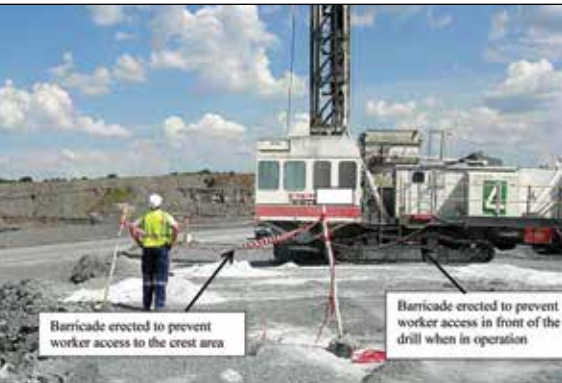
Figure 8: Barricade erected to prevent worker access to the crest area and in front of the drill when it is in operation. Note that the chevron tape has since been replaced with medium weight rope.
