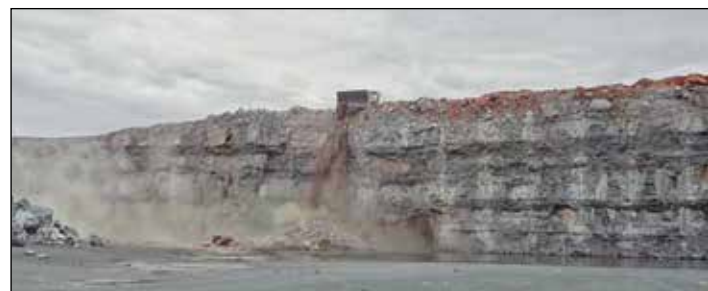
Figure 6: A front-end loader pushing waste overburden over a crest onto the orebody below.
