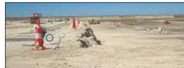
Figure 13: A text book example of a barricade that prevents access to the crest and is easy to erect and dismantle.
