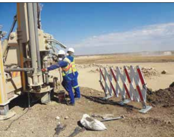
Figure 10: Drilling with a portable barricade can be cumbersome.
