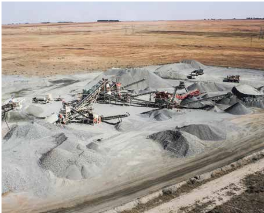
A view of the secondary crushing plant at the B&E International crushing site at Kusile.
