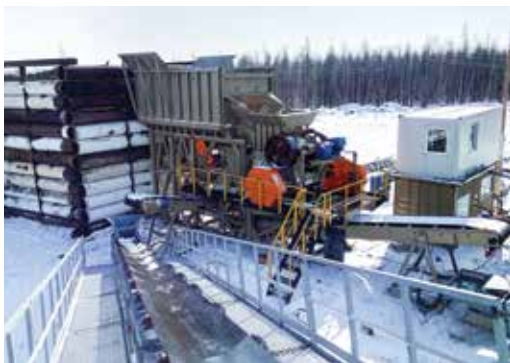
The full modular plant at the Al Rosa facility offers primary and secondary crushing and screening capabilities.
