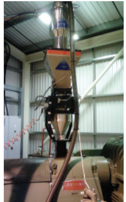
○ Maguire loss-in-weight (LIW) hopper installed at the Prysmian plant
